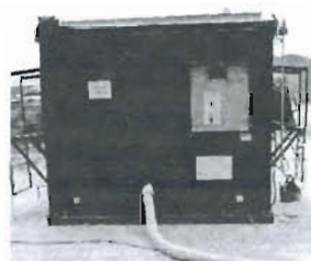
Conveying Equipment: Saw dust is conveyed through metering system.
