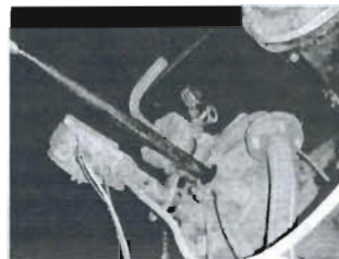
Burner Pipe: Saw dust is conveyed through a port specially designed for alternative fuels.
