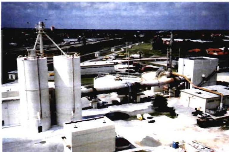
Figure 3-1 Alexander Orr, Jr. WTP Lime Recovery Plant
