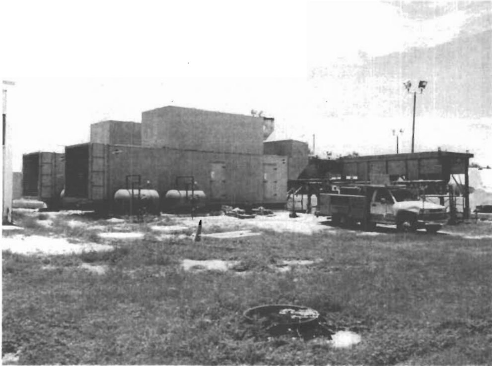
Above: New EMD Nos. 4 and 5, west side view Picture taken: 7/3/2006 12:18:08 (from header information embedded in image)
