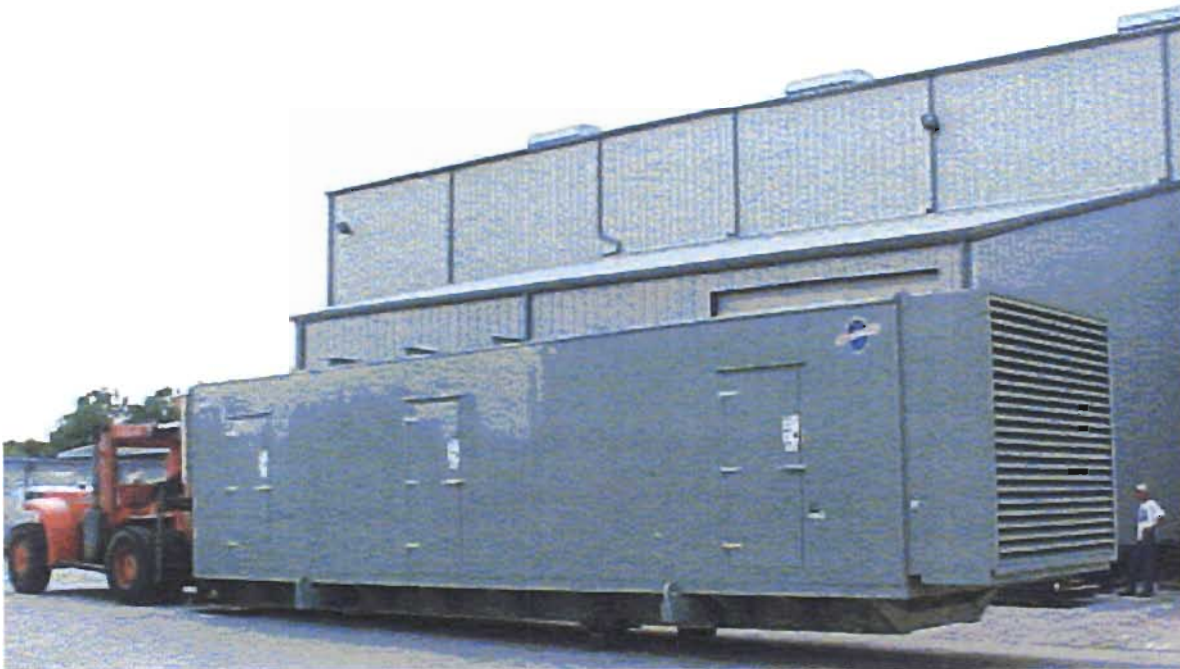
Figure 3-3 - EMD Model 20F4B Unit and Enclosure at Stewart & Steven's Texas Facility
