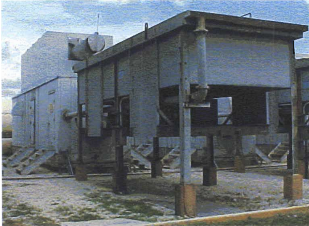
Figure 3-2 - EMD Model 20-645F4B Unit with External Radiator
