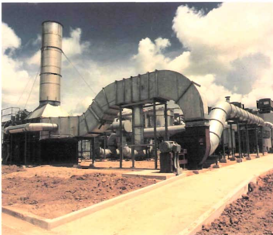
Catalytic incineration occurs via a platinum metal catalyst
