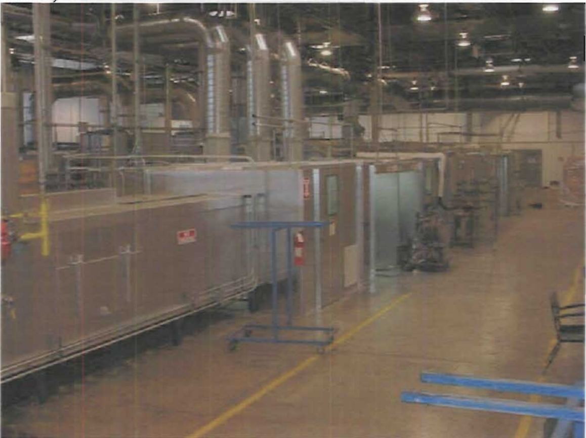
Paint line No.1 showing enclosed conveyors and ductwork that routes emissions to the RTO.
