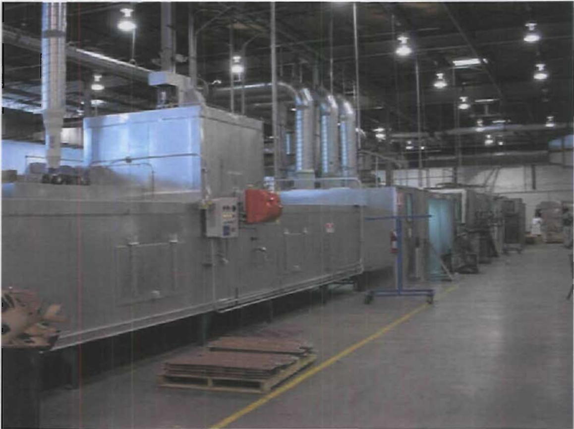
Paint Line No. 1 showing enclosed conveyors and new gas oven (enclosure with red controls).
