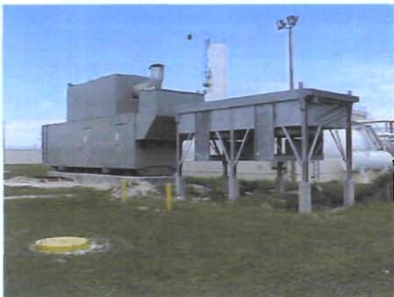
Figure 3-2 EMD 20-645F4B (South District WWTP)
