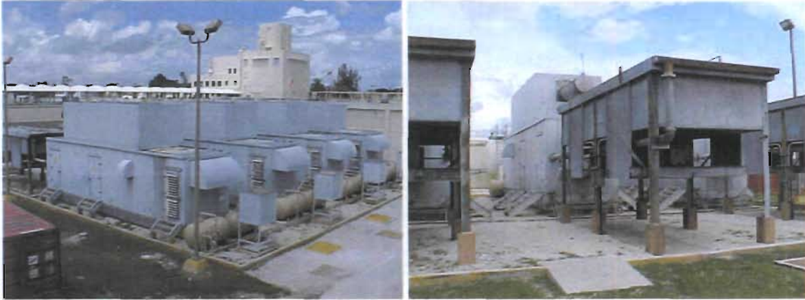
Figure 3-3 Existing Standby Generator Bank (Alexander Orr, Jr. WTP)
