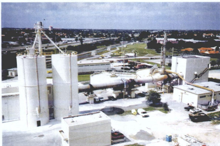
Figure 3-1 Alexander Orr, Jr. WTP Lime Recovery Plant
