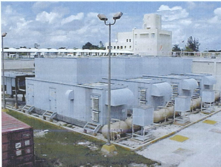
Figure 3-2 Alexander Orr, Jr. WTP Standby Generator Bank
