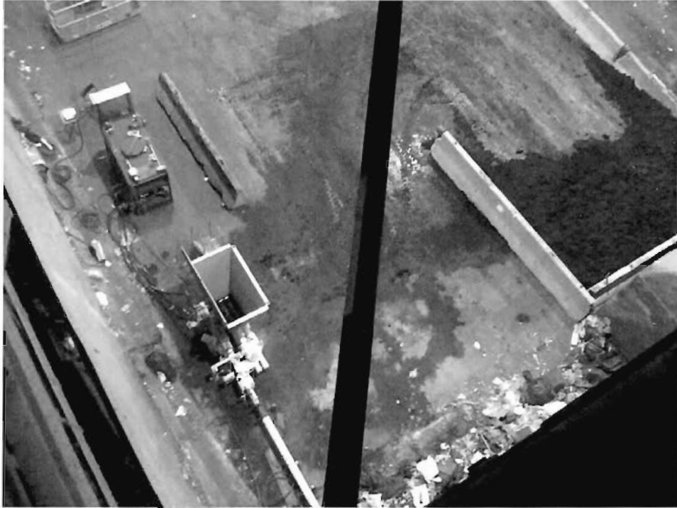
Figure 12 – Overhead View of Storage and Feed Equipment
