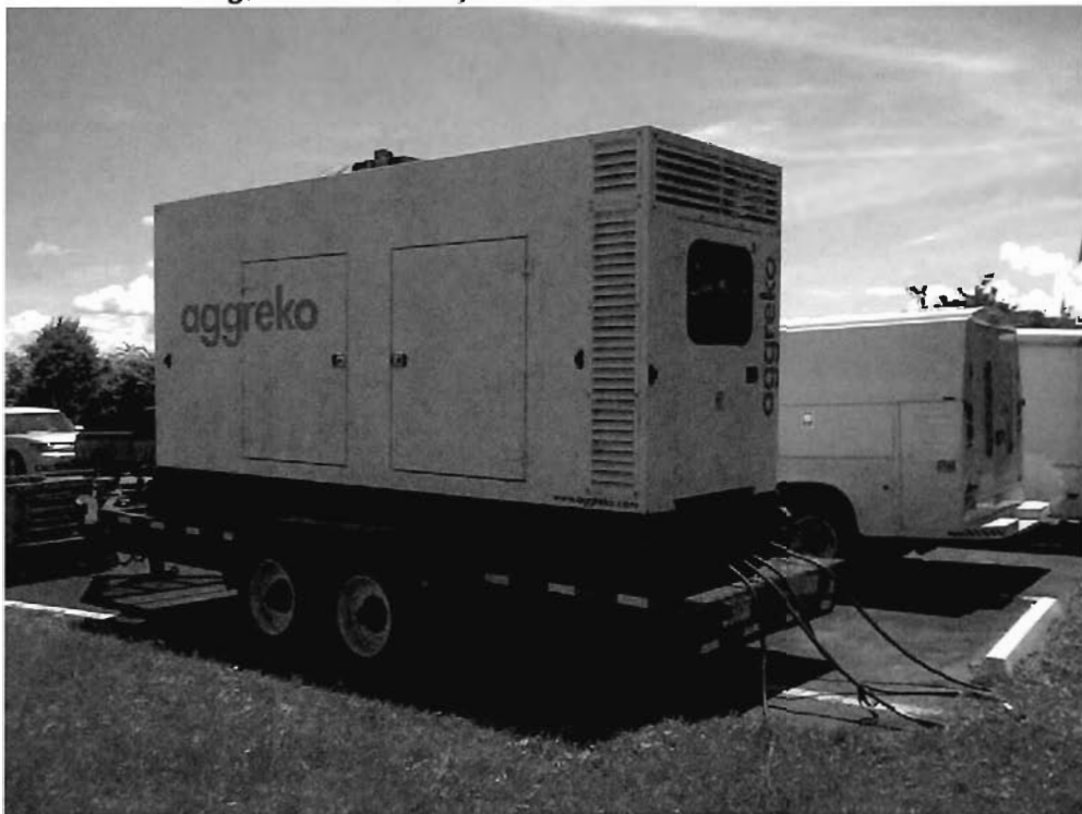
Figure 8 – 480V/200 Amp Generator
