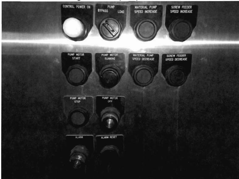
Figure 10 – Screw/Pump Manual Controls
