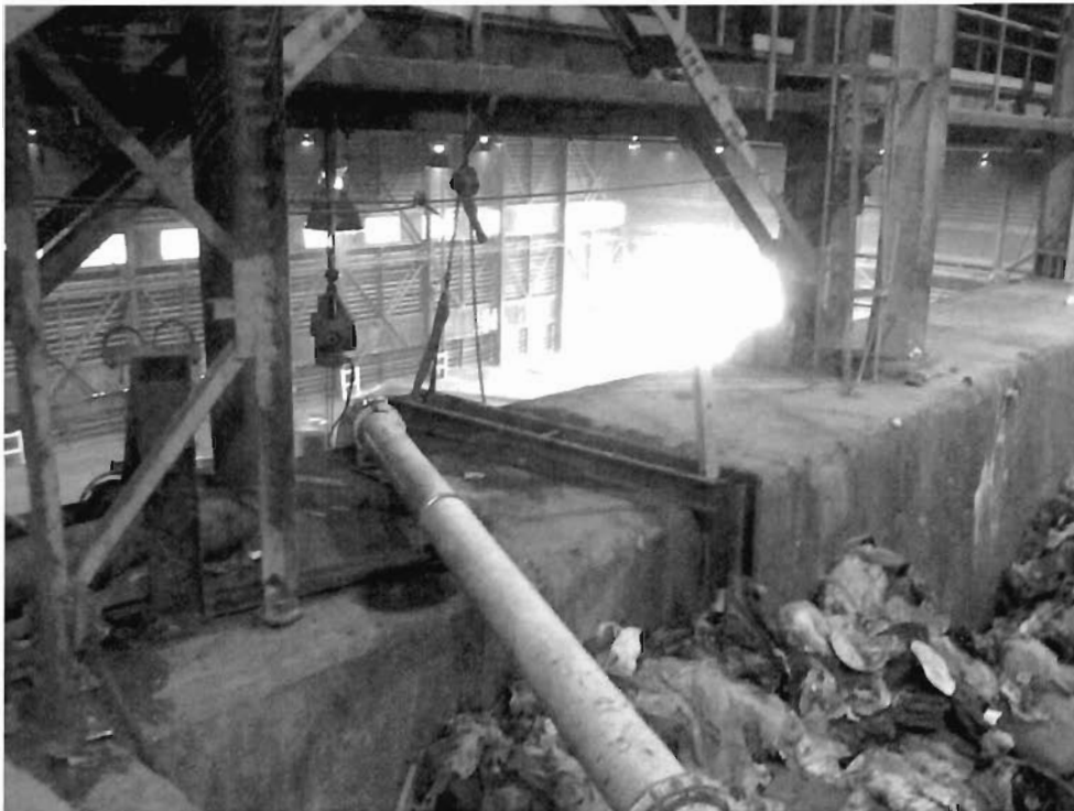
Figure 14 – Piping from Tipping Floor
