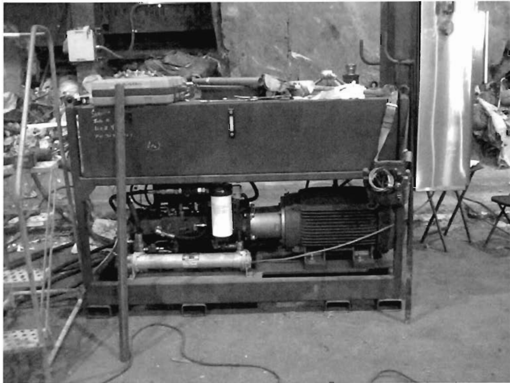
Figure 7 - 100 HP Hydraulic Power Unit and Control Panel
