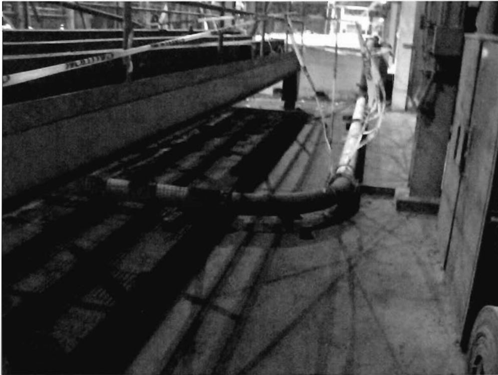
Figure 16 – Piping to Charging Hopper
