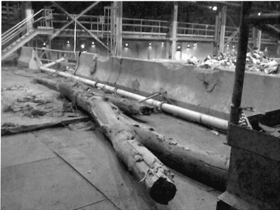
Figure 15 – Piping at Charging Hopper Level North of Refuse Pit
