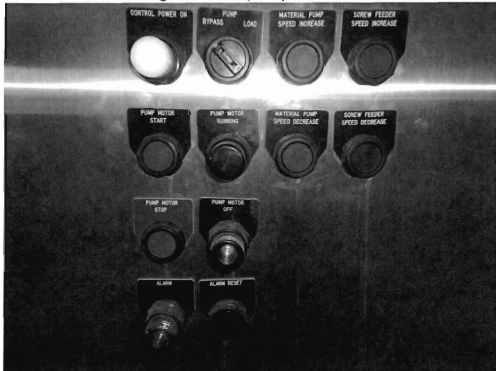
Figure 10 – Screw/Pump Manual Controls
