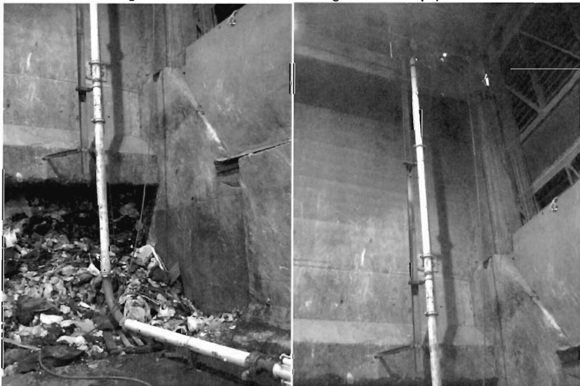
Figure 13 – Piping to Charging Hopper Level
