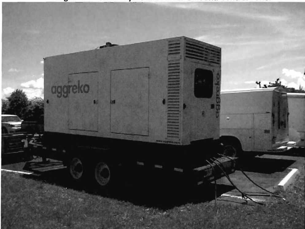
Figure 8 – 480V/200 Amp Generator
