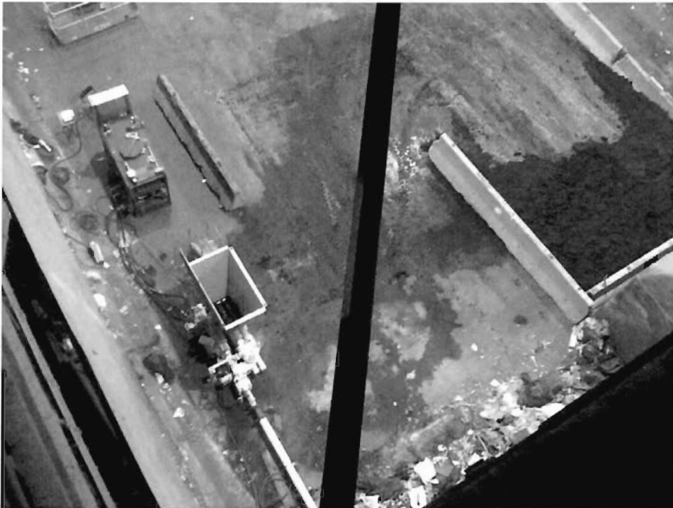
Figure 12 – Overhead View of Storage and Feed Equipment
