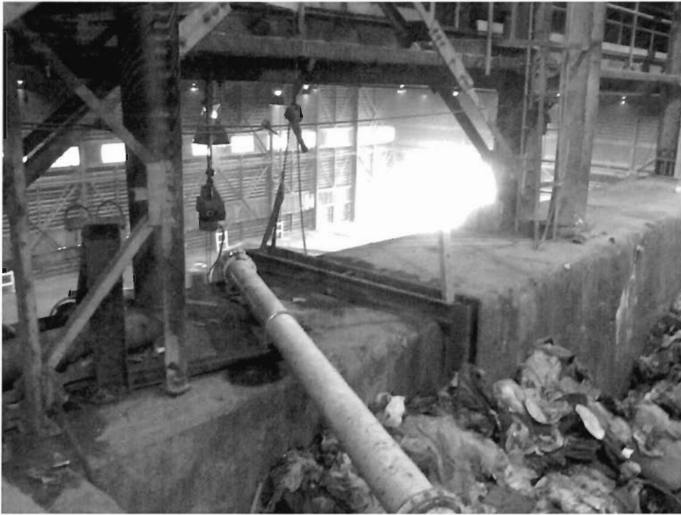
Figure 14 – Piping from Tipping Floor
