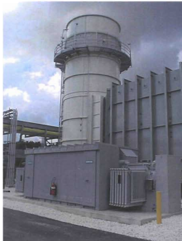
Combustion Turbine Stack
