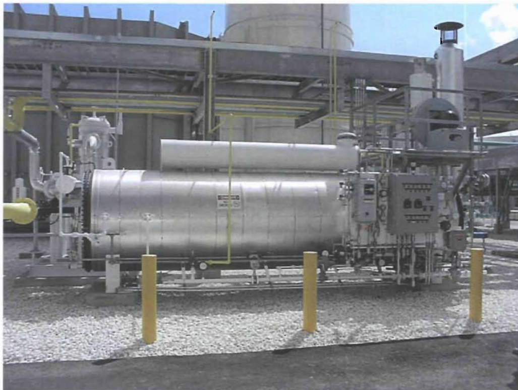
Fuel Gas Heater
