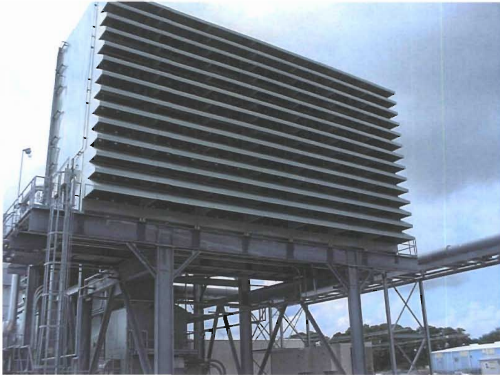
Combustion Turbine Air Inlet
