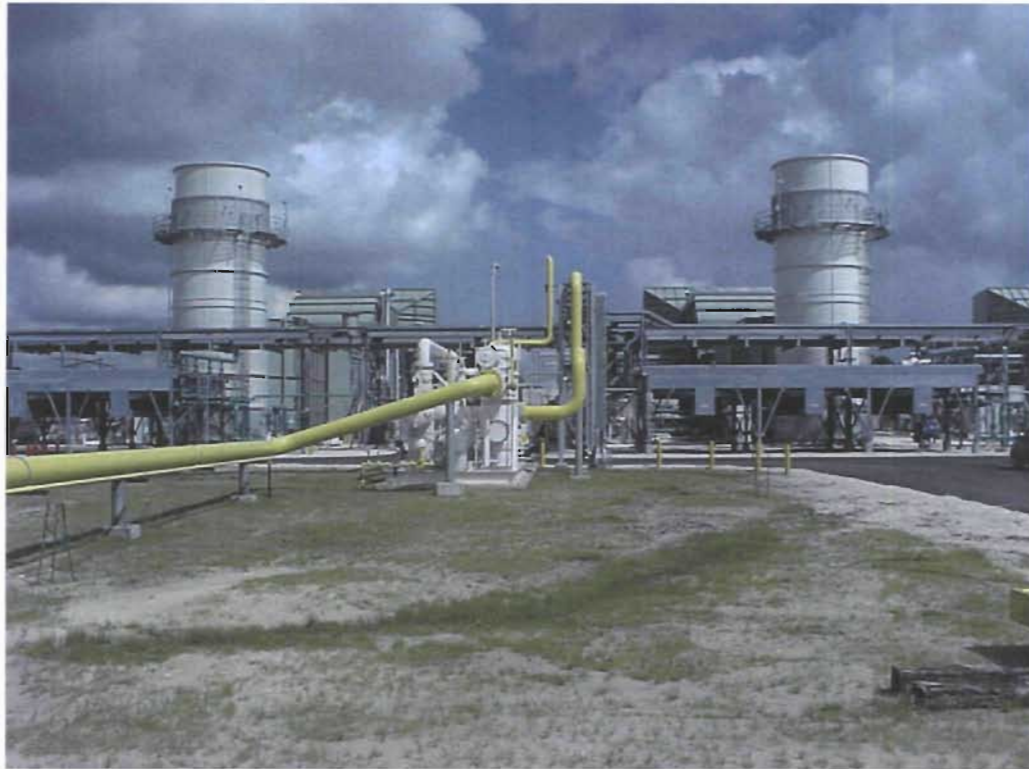
Front View - Combustion Turbine and Natural Gas Fuel Line
