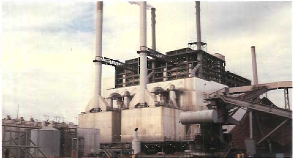
Two 370,000 ACFM wet bottom, precipitators — Mansfield, Louisiana.
