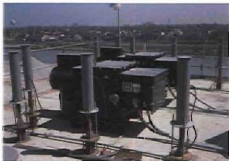
Single bushing, side mounted, transformer rectifier with CLR
