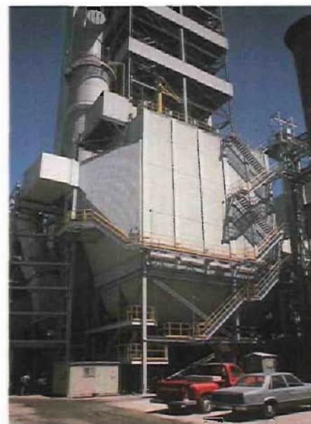
Alkali bypass preheater precipitator — Davenport, California.
