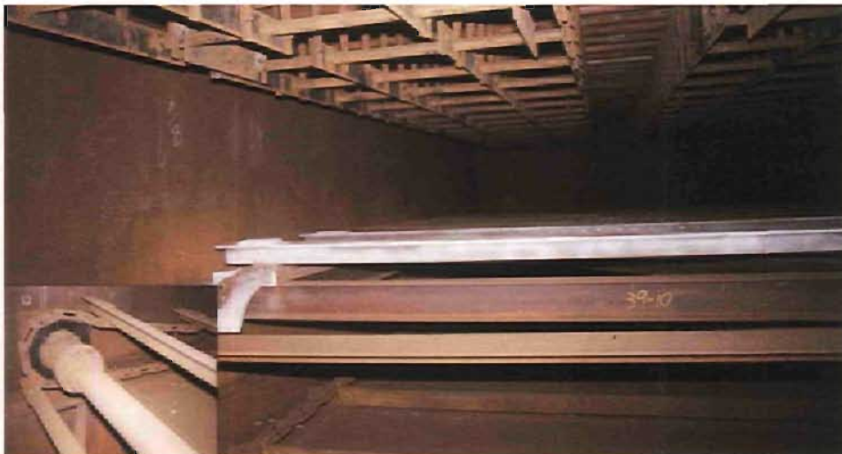
Typical heavy duty drag scraper conveyor system.
