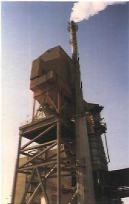
A 650 TPD Sludge Lime Kiln Precipitator followed by a wet scrubber — Brunswick, Georgia.
