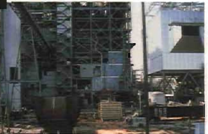
► ESP's erected in remote location.
