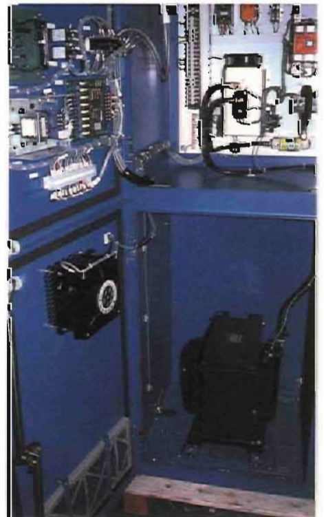
Single Console with Current Limiting Reactor
