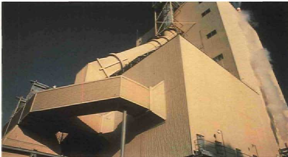
One 2-chamber, wet bottom, low odor recovery boiler precipitator, with truncated outlet nozzles, designed for 730,400 ACFM — Crossett, Arkansas.
