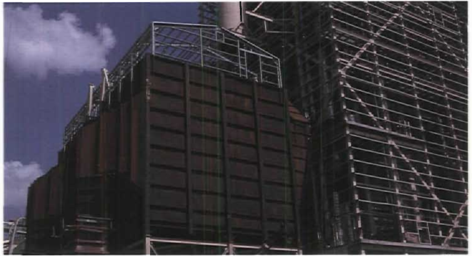
Two single chamber dry bottom precipitators on a 470,000 ACFM low odor recovery boiler — Brunswick, Georgia.
