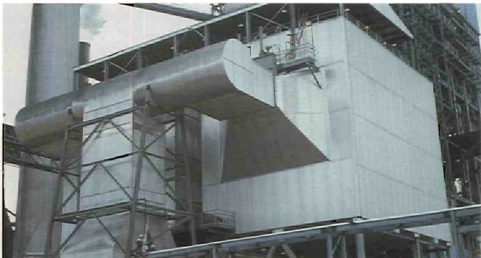
Two single chamber 440,000 ACFM dry bottom low odor recovery boiler precipitators — Deridder, Louisiana.
