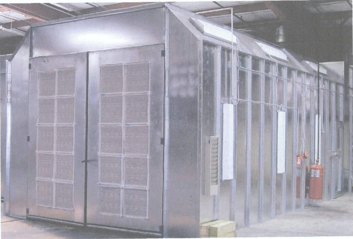
Spray Booth with Fire Suppression
