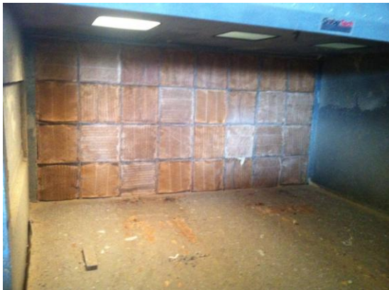
New filters installed on 7/28/13.
