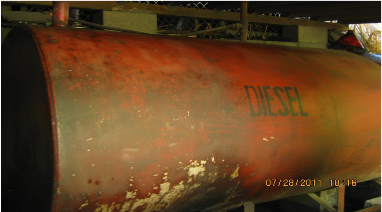
DIESEL FUEL TANK
