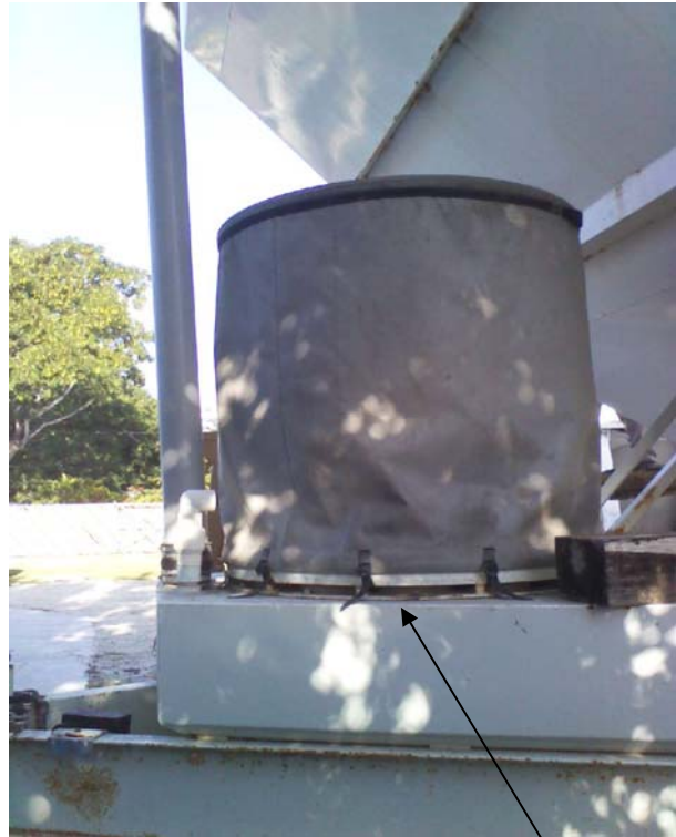
Baghouse; emissions, if any, would exit around the bottom
