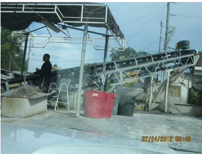
Photo ID No: IMG_460 – Oversize Return Belt No. 2 back to crusher hopper. There is a noticeable windshield glare in this image.
