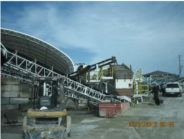
Photo ID No: IMG_464 – Screen No. 3 with view full view of Pile Conveyor No. 1
