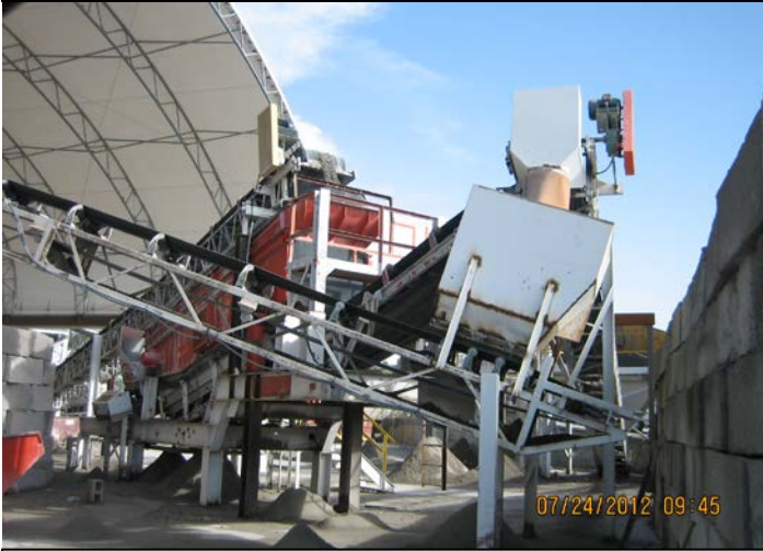
Photo ID No: IMG_465 – Pile Conveyor 1 and Pile Conveyor 2 drop points with Hopper No. 2 in background.
