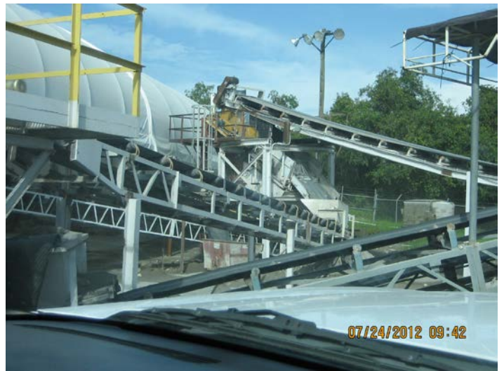
Photo ID No: IMG_461 - Non-Metallic Mineral Processing Plant Screen No. 1(color: Orange) operation in progress.
