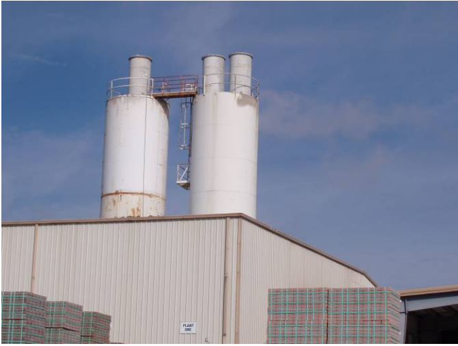
Photo ID No: 1050372_Photo_01_24_2012-4 Time: Approx. 10:30 AM. Close-up photo of the two silos for Plant 1 (EU001, EU002, and EU003), camera facing approx. NNW.
