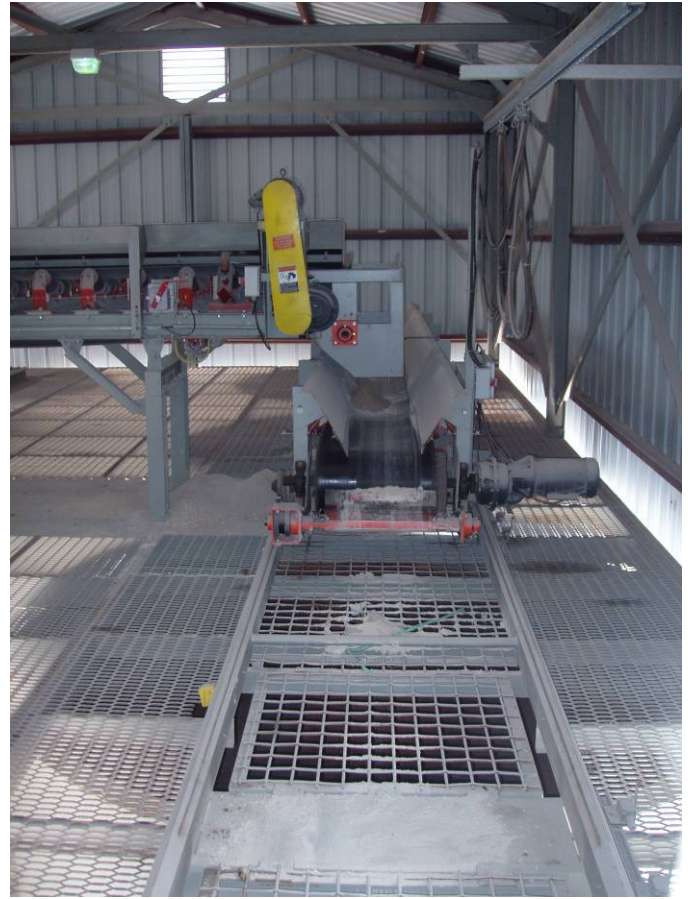
Photo ID No: 1050372_Photo_01_24_2012-36 Time: Approx. 12:40 PM Inside the structure on top of the storage bins in Plant 4, where aggregate materials are loaded. The grates are directly on top of each storage bin. Camera is facing approx. W.
