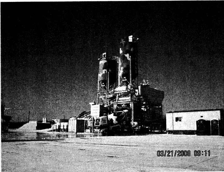
Photo ID No. / Date / Time: Inland Mat 032108 (6) – Left to right: flyash silo, cement silo, weigh hopper
