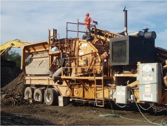
Photo ID No: 7775229_Photo_9_of_11_on_09_27_2012; Date: 09/27/2012; Time: Approx. 08:30 AM. Close-up of crusher and crusher engine. Man is standing above crusher compartment. Closer to the foreground of the photograph is the crusher engine, which looks like a black box with a small stack. The camera is facing approx. SW.
