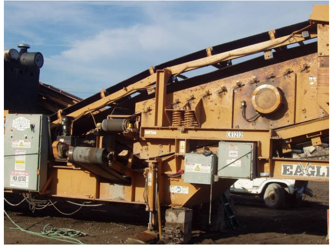
Photo ID No: 7775229_Photo_11_of_11_on_09_27_2012; Date: 09/27/2012; Time: Approx. 08:30 AM. Close-up of right side (East side) of screener (front side assumed to be exit of screener). The camera is facing approx. SW.
