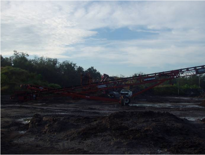
Photo ID No: 7775229_Photo_5_of_11_on_09_27_2012; Date: 09/27/2012; Time: Approx. 08:30 AM. View of conveyor belt to product pile (pile not visible). The camera is facing approx. S.
