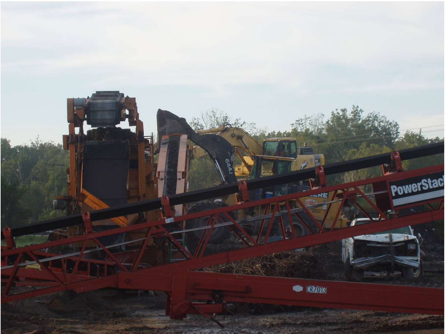
Photo ID No: 7775229_Photo_3_of_11_on_09_27_2012; Date: 09/27/2012; Time: Approx. 08:30 AM. Crushing operation. The camera is facing approx. S. In the background is the excavator, which loosens up the material to be crushed so that the front-end loader, also visible in the background, can load the crusher hopper. From the screener exit (visible with magnetic belt on top), the product drops to one conveyor belt (barely visible in photograph), then drops onto the conveyor belt (foreground) that leads to the product pile (not visible).
