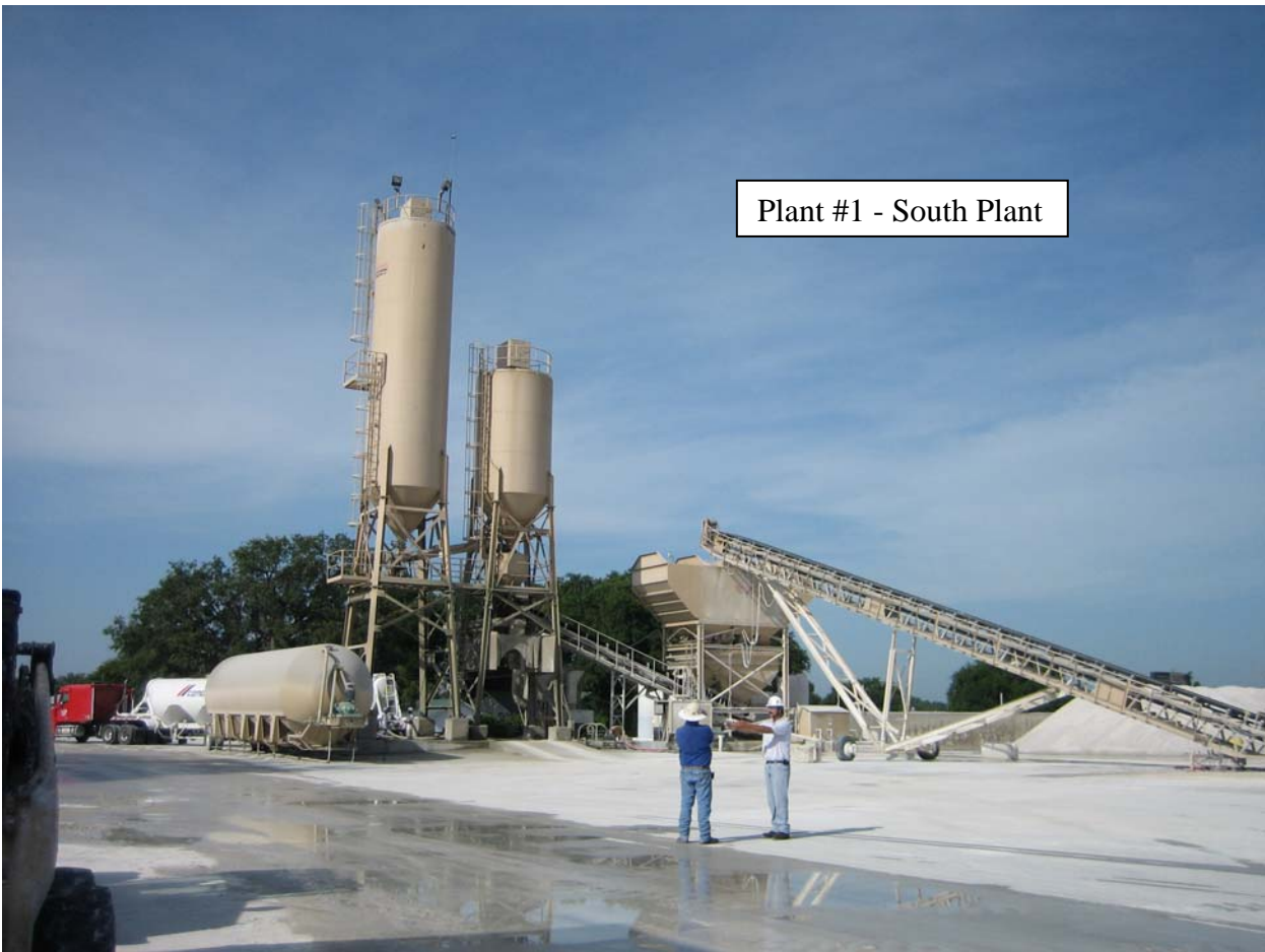
Emission Unit #4 Truck Load Out Recovery System --Plant #1-South Plant
