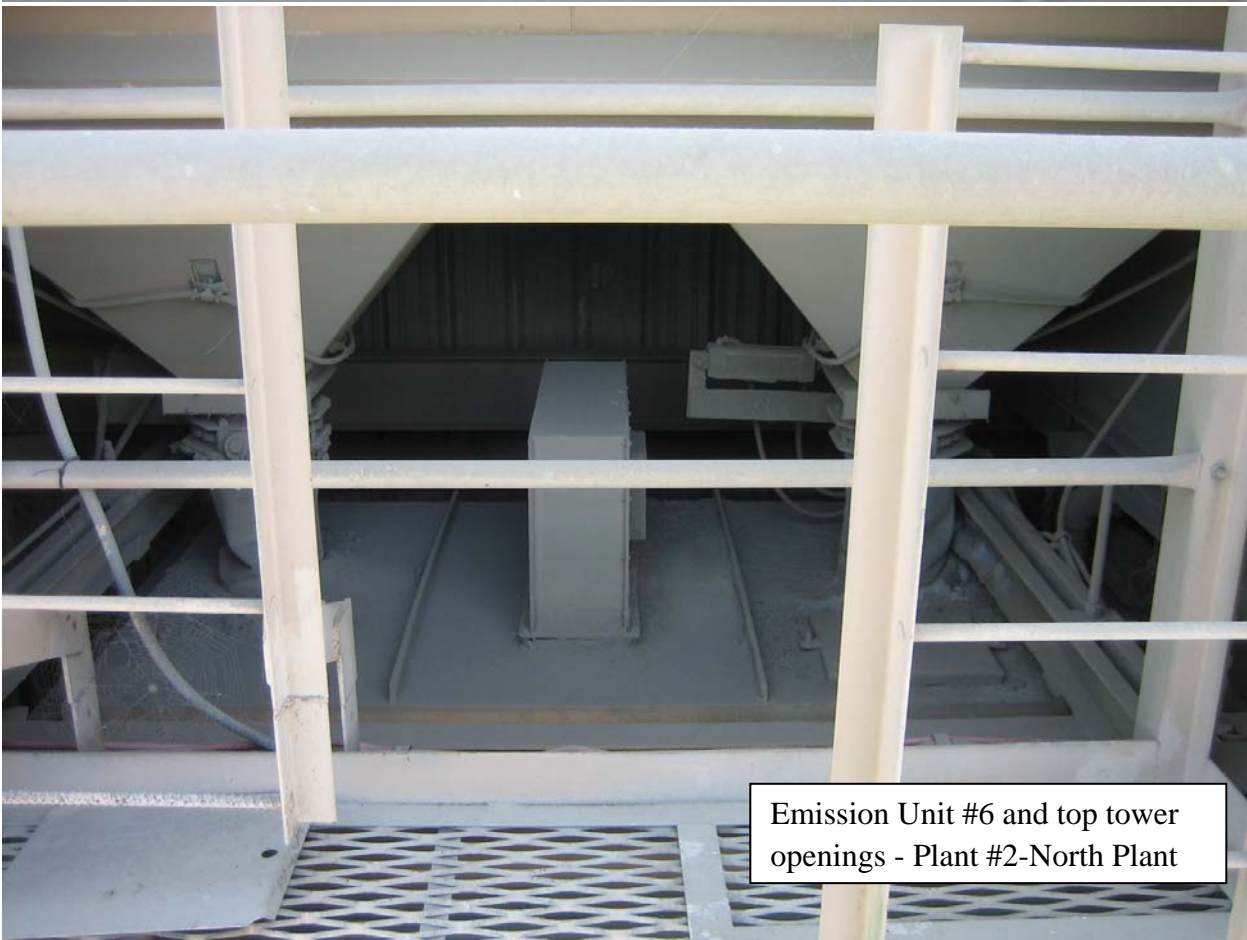
Emission Unit #6 middle and top tower openings - Plant #2-North Plant
