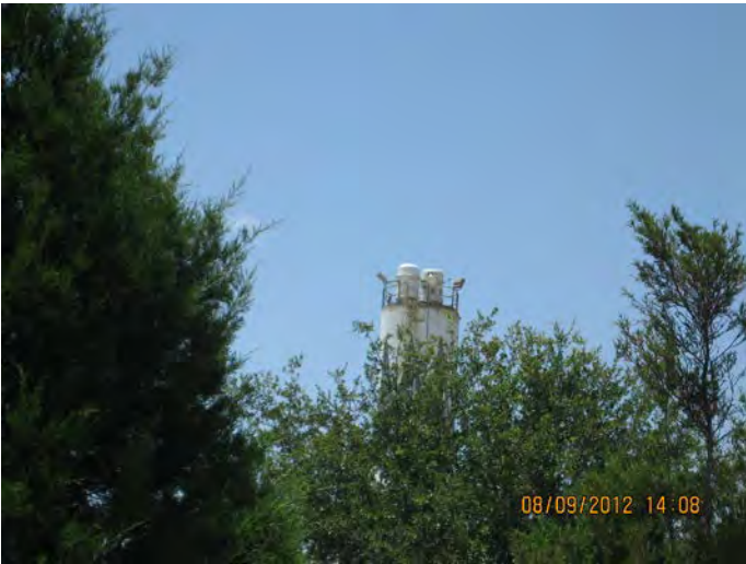
Photo ID No: IMG_426 - B. E. T. ER Mix, Inc. Zephyrhills Plant silo top dust collectors. Evidence of Flyash on silo top.
