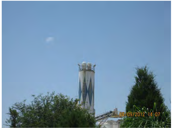
Photo ID No: IMG_425 - 2 silo top dust collectors (Emission Unit Nos. 002 and 003) close-up view from MOMHP.
