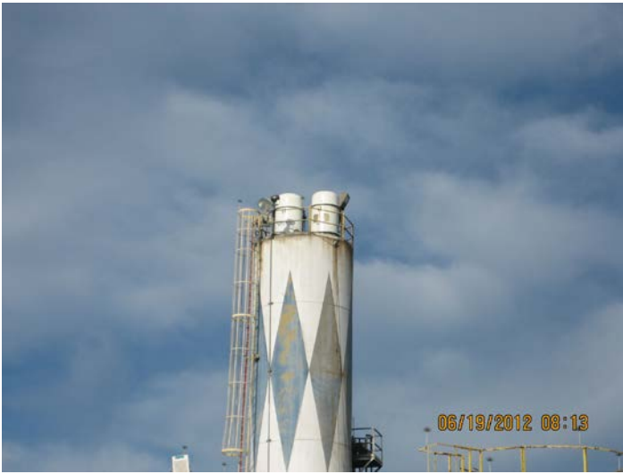
Photo ID No: IMG_487 – Close-up view of 2 new silo top dust collectors. Emission Unit No. 002 (Cement side) on left and Emission Unit No. 003 (Flyash side) on the right.
