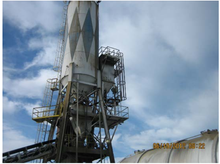
Photo ID No: IMG_489 – Close-up view of CDC (Emission Unit No. 004) which controls the truck load out and the weigh hopper.
