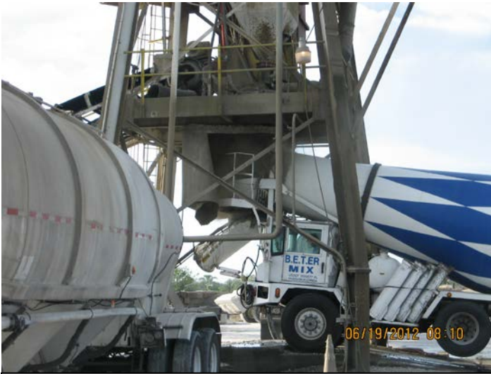
Photo ID No: IMG_482 – B. E. T. ER Mix, Inc. Zephyrhills Plant truck loading activity
