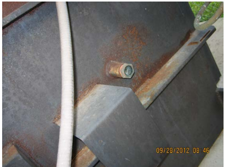
Photo ID No: IMG_441 – This photo shows the flame view port on the back of the cremation unit.
