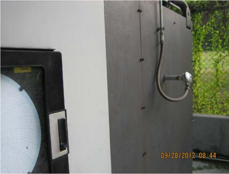
Photo ID No: IMG_438 – Photo shows secondary chamber thermocouple placement on the right side of the cremation unit.
