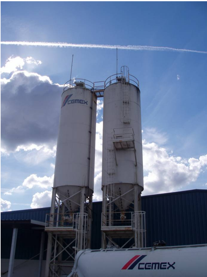
Photo ID No: 1050350_Photo_01_24_2012-15 Time: Approx 14:25 PM View of both the North silo (EU006) and the South silo (EU005), camera facing approx. W.
