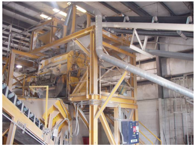
Photo ID No: 1050350_Photo_01_24_2012-12 Time: Approx 14:20 PM Weighing and batching operations located inside the building at the facility; camera facing approx. NE. Silos are outside the building, just behind this equipment.
