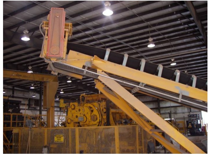
Photo ID No: 1050350_Photo_01_24_2012-14 Time: Approx 14:20 PM Top of the conveyor belt that is part of the weighing and batching equipment inside the building at the facility; camera facing approx. NW.
