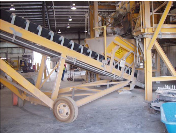
Photo ID No: 1050350_Photo_01_24_2012-13 Time: Approx 14:20 PM Conveyor belt that is part of the weighing and batching equipment inside the building at the facility; camera facing approx. N.
