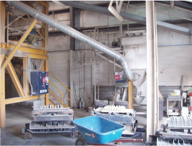
Photo ID No: 1050350_Photo_01_24_2012-11 Time: Approx 14:20 PM Some weighing and batching equipment located inside the building at the facility; camera facing approx. ENE.
