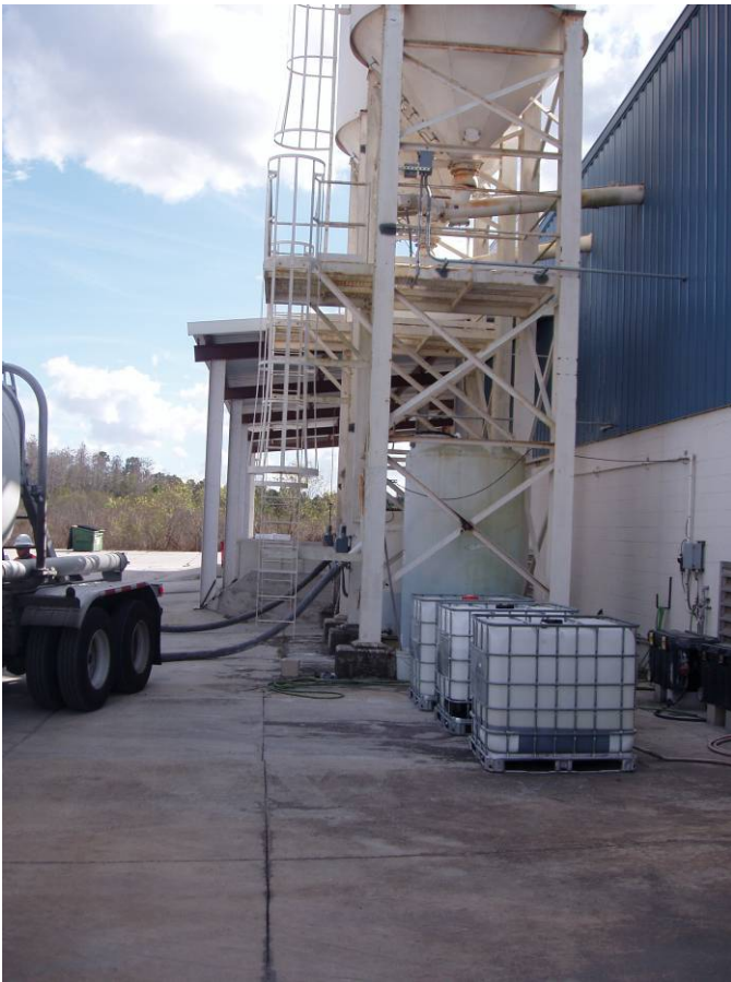
Photo ID No: 1050350_Photo_01_24_2012-1 Time: Approx. 13:40 PM The North silo (front silo in photo) is EU006, also listed as silo #2, and was filled with white cement. The South silo (back silo in photo) is EU005, also listed as silo #1, and was filled with grey cement. Camera facing approx. S.
