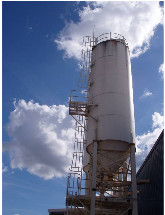
Photo ID No: 1050350_Photo_01_24_2012-3 Time: Approx. 13:40 PM View of North silo (EU006) with South silo (EU005) behind. Camera facing approx. S.
