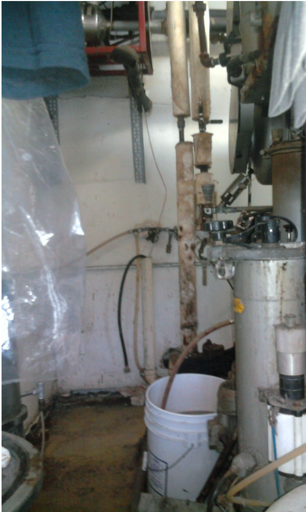
Photo ID No. 01 Wednesday, April 04, 2012, 10:42:58 AM Water collection bucket uncovered.
