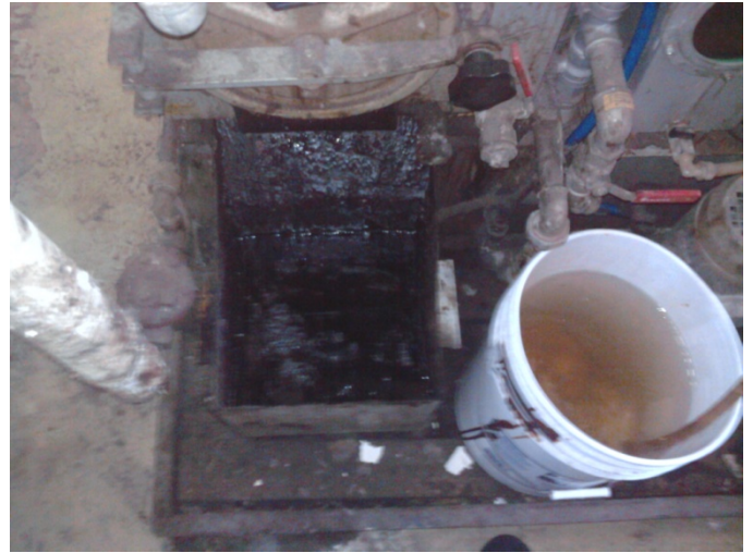
Photo ID No.02 Wednesday, April 04, 2012, 10:43:28 AM Condensation collector in working order, uncovered condenser water bucket.
