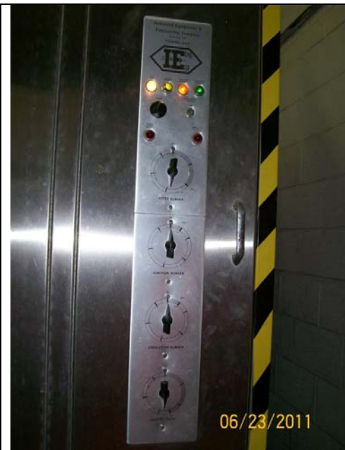
Control panel, close-up in next photo frame
