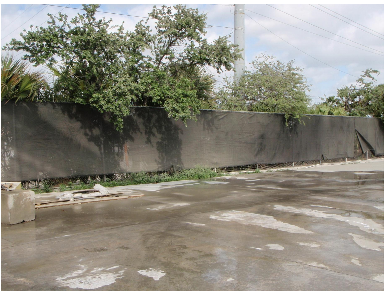
Cement dust on the plants from the initial release. The facility has water the ground to reduce the dust.
