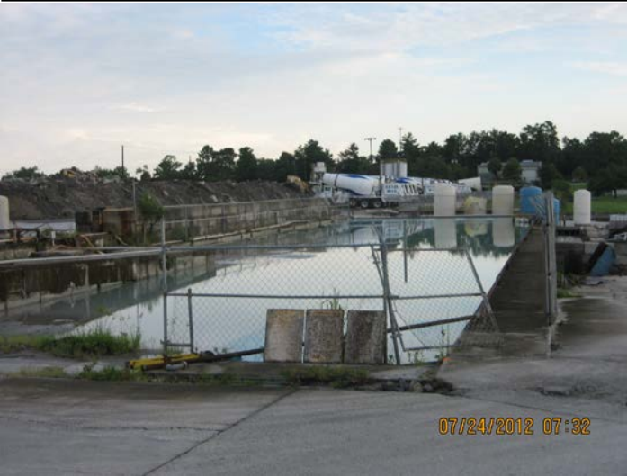
Photo ID No: IMG _438 – This photo shows a closer view of the wastewater pond.
