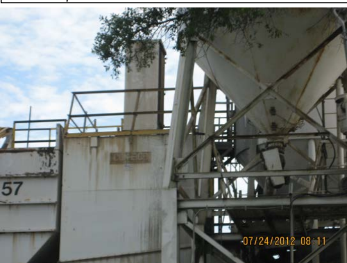
Photo ID No: IMG _442 – This photo shows a closer view of silo dust collector for small silo (Emission Unit No. 004)
