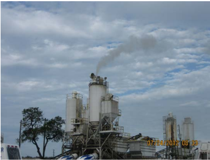
Photo ID No: IMG_447 – This photo shows flyash release from new dust collector for Emission Unit No. 11. This release quickly dissipated and lasted less than 6 minutes.
