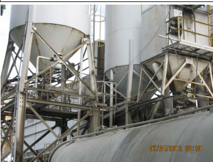
Photo ID No: IMG _441 – This photo shows silo dust collector for small silo (Emission Unit No. 004)
