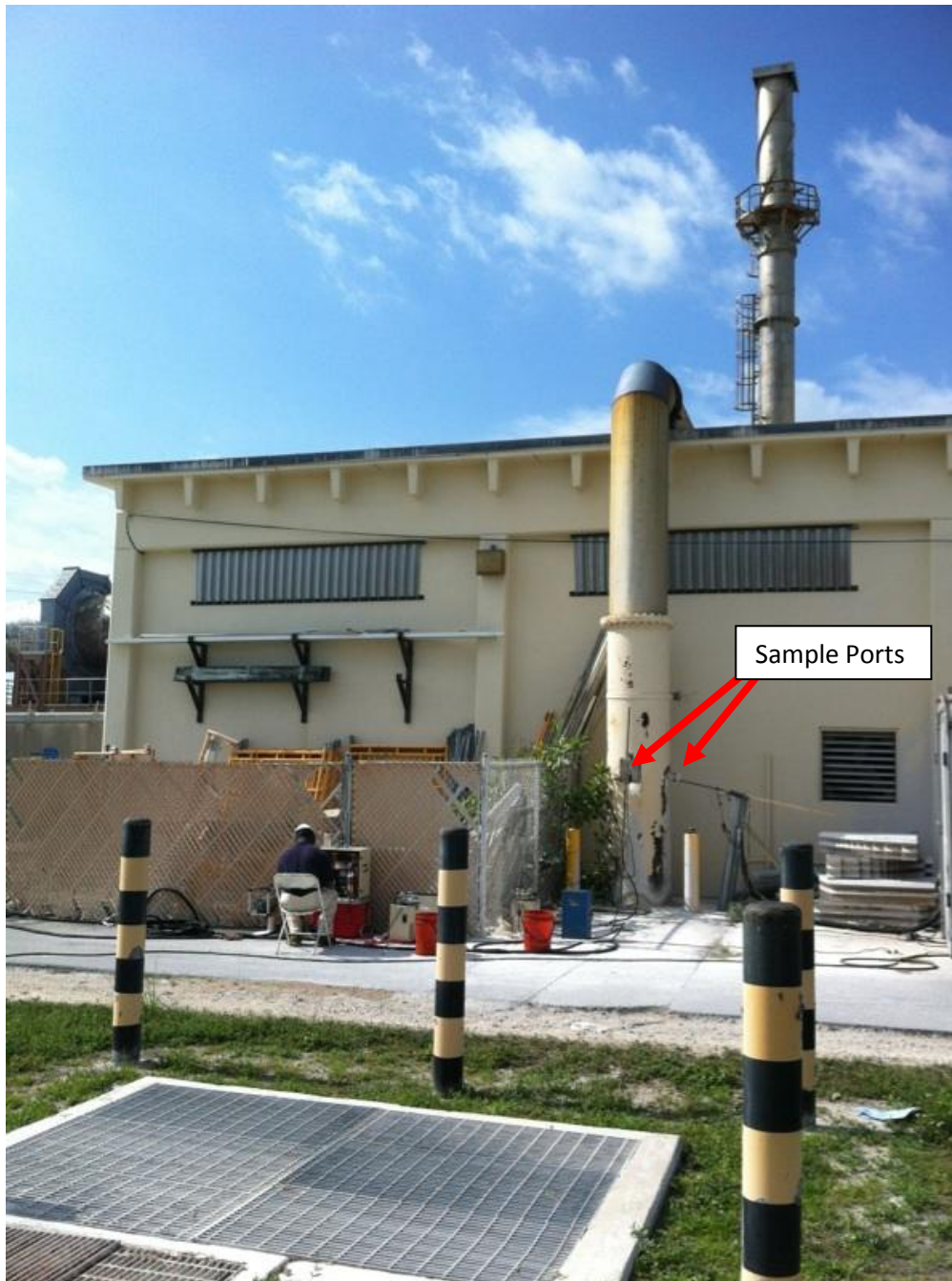
Location of Stack Test. Note direction of gas flow is down. (Stack in background is blocked and inoperable.)
