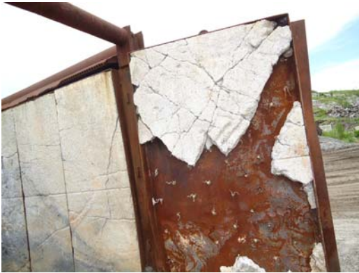
Inside of entrance door to Mobile Air Curtain Incinerator (ACI).
