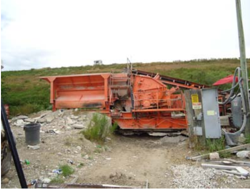
Existing stationery crusher unit with adjacent electrical supply (7775112).
