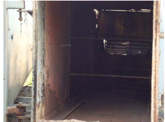
Inside of ACI unit.
