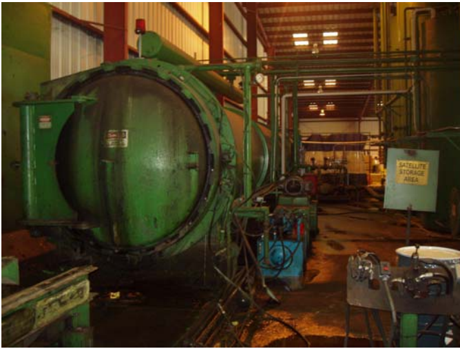
Photo ID No: 1190048_Photo_03_01_2012-003 Time: Approx. 10:00 AM Front view of the horizontal cylinder for preserving wood products with CCA. The camera is facing approx. N.
