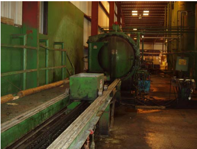
Photo ID No: 1190048_Photo_03_01_2012-006 Time: Approx. 10:00 AM View of small rail system used to load wood products into horizontal cylinder for CCA treatment. The camera is facing approx. N.
