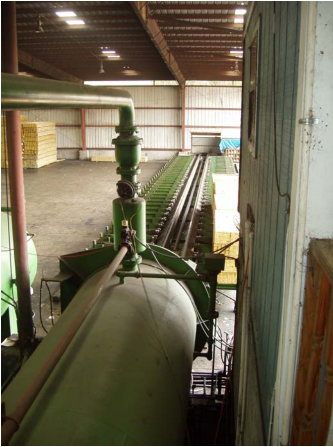
Photo ID No: 1190048_Photo_03_01_2012-017 Time: Approx. 10:30 AM View from control room for cylinders 1 and 2. The camera is facing approx. E.
