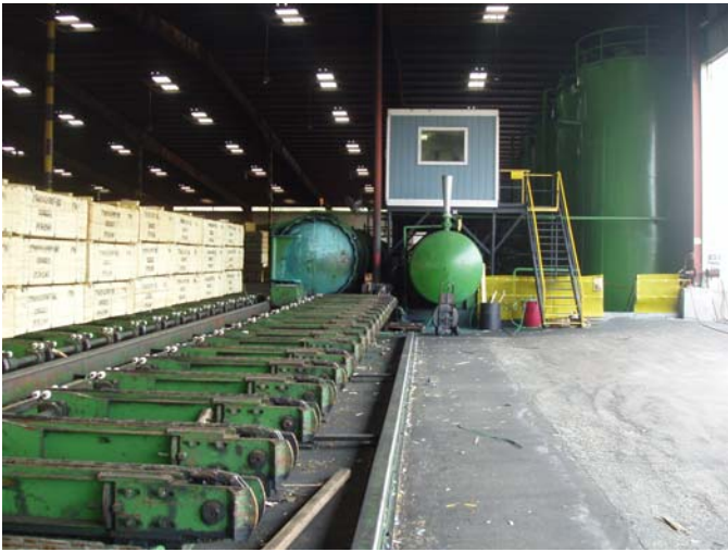
Photo ID No: 1190048_Photo_03_01_2012-010 Time: Approx. 10:30 AM Horizontal cylinders (cylinders 1 and 2) for pressure treating wood products with chemicals such as micronized copper azole (MCA), boron, and alkaline copper quat (ACQ). CCA is not used in these cylinders. Wood products are loaded and unloaded using the loading track visible in the photo. The camera is facing approx. E.
