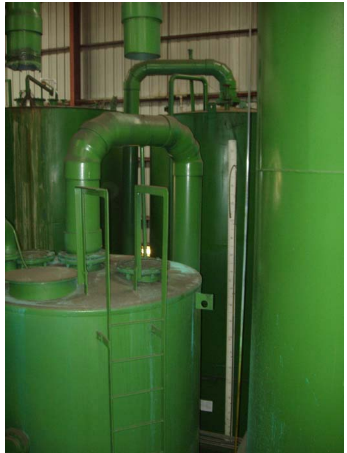
Photo ID No: 1190048_Photo_03_01_2012-013 Time: Approx. 10:30 AM Tanks used for storing and preparing chemicals. The camera is facing approx SE.
