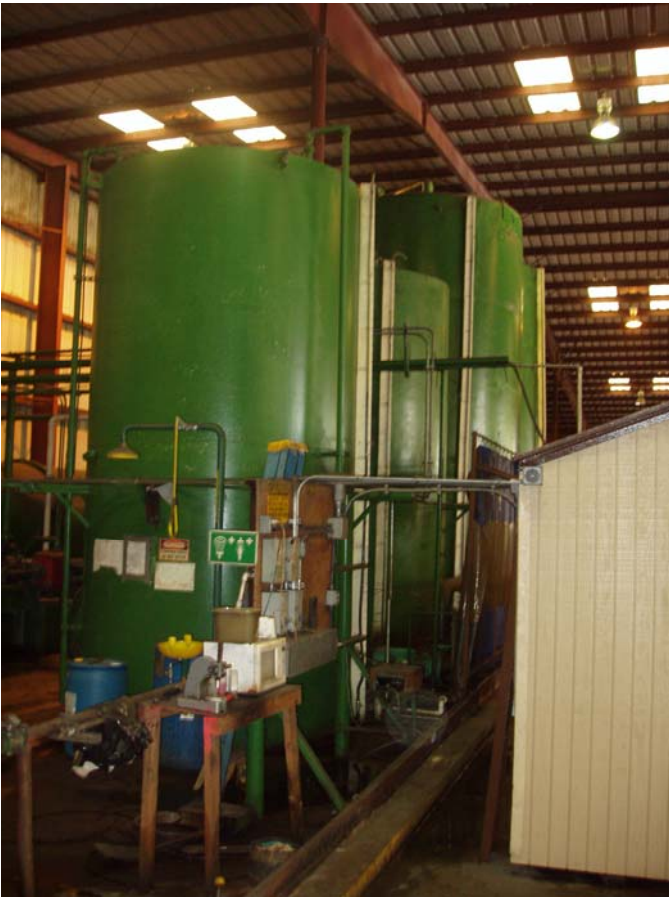
Photo ID No: 1190048_Photo_03_01_2012-001 Time: Approx. 10:00 AM Tanks for preparing chromated copper arsenate (CCA) for wood preserving. The camera is facing approx. NW.
