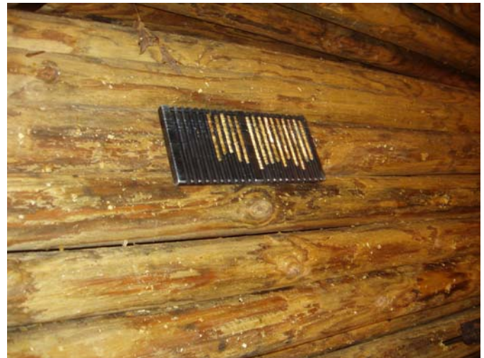
Photo ID No: 1190048_Photo_03_01_2012-009 Time: Approx. 10:15 AM Drill samples of pressure treated wood pack. The drill samples are taken to determine the depth of penetration of preservative chemical, which in this case is CCA. For individual wood products with a diameter, or thickness, of less than or equal to 4" (inches), the penetration depth of preservative must be at least 1.75", and for a thickness of greater than or equal to 6", the penetration depth must be at least 2.50".
