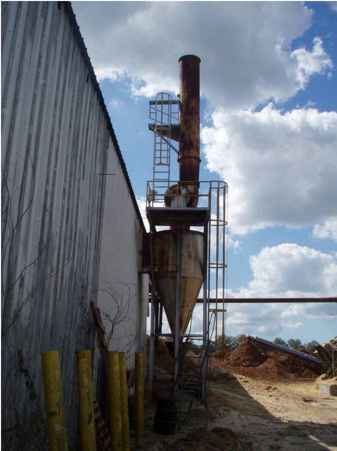
Photo ID No: 1190011_Photo_03_01_2012-006 Time: Approx. 14:00 Stack from ABCO Boiler. The ABCO boiler was being repaired during the inspection and was not operating. The stack is located on the North side of the building that houses the Hurst and ABCO boilers. The camera is facing approx. W.
