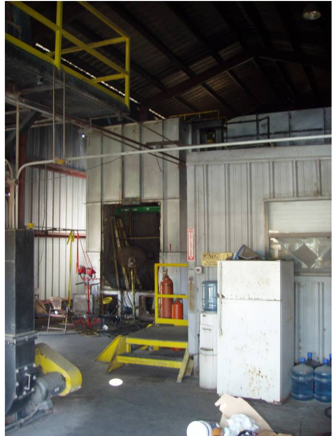
Photo ID No: 1190011_Photo_03_01_2012-007 Time: Approx. 14:00 View of the ABCO boiler and control room for the Hurst and ABCO boilers. The yellow steps lead to the control room. During the site inspection, the ABCO Boiler was in the process of being repaired. In the photograph, the ABCO boiler is the structure with an opening, next to two red tanks. The camera is facing approx. SW.
