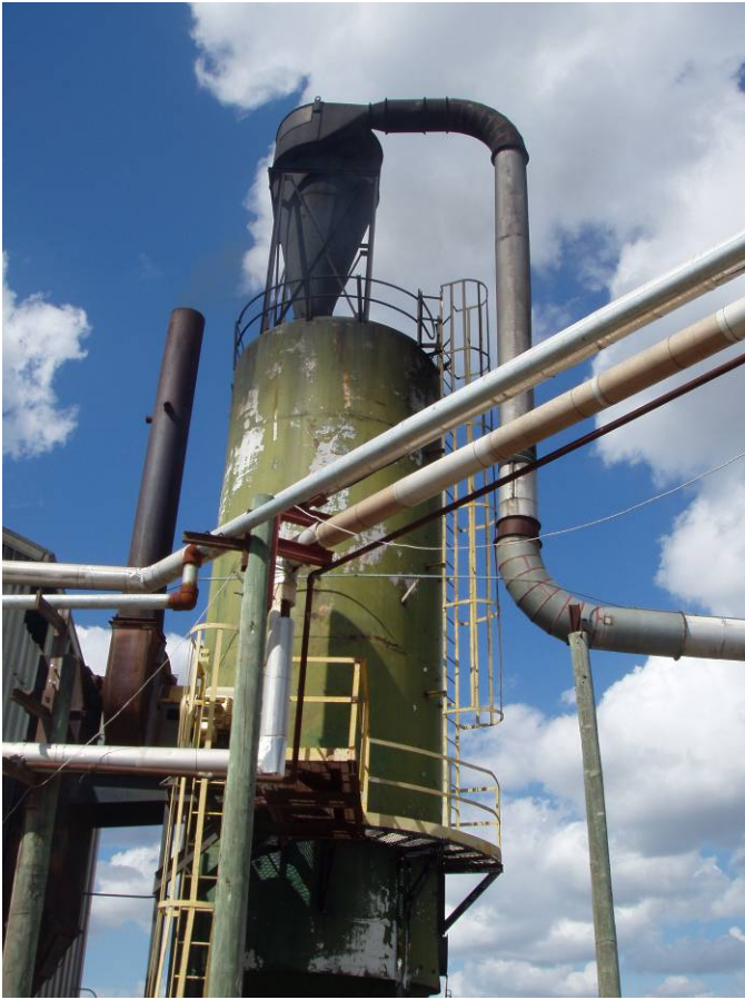
Photo ID No: 1190011_Photo_03_01_2012-008 Time: Approx. 14:15 South face of the sawdust storage silo (green) for the Hurst Boiler and the stack (brown/black) from the Hurst boiler. Pipe lines carry sawdust generated from woodworking operations to the cyclone on top of the sawdust storage silo. The cyclone controls particulate matter emissions from the sawdust storage and transfer operations. Steam generated from the Hurst boiler travels in pipe lines to the kilns, and these steam lines are visible in the foreground of this photograph. The camera is facing approx. N.
