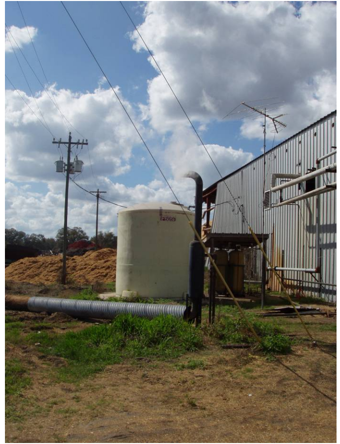
Photo ID No: 1190011_Photo_03_01_2012-009 Time: Approx. 14:15 Blowdown pipe for #####. Camera is facing approx. W.
