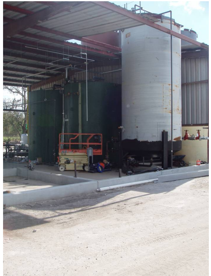
Photo ID No: 1190011_Photo_03_01_2012-017 Time: Approx. 14:45 Construction operations for lumber pressure treatment facility on site of Robbins Manufacturing Co. in Tarrytown, FL (Sumter County). This construction operation does not currently have an air construction permit.
