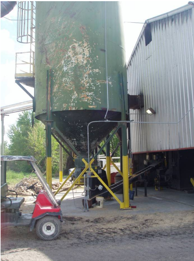
Photo ID No: 1190011_Photo_03_01_2012-004 Time: Approx. 14:00 Sawdust storage silo with auger below to transport sawdust for combustion in the Hurst Boiler. The camera is facing approx. S.
