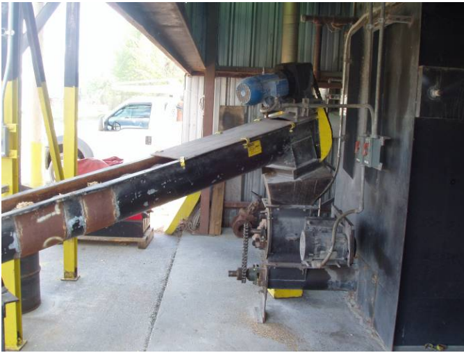
Photo ID No: 1190011_Photo_03_01_2012-003 Time: Approx. 13:45 Auger transporting sawdust for combustion in the Hurst Boiler. The camera is facing approx. S.
