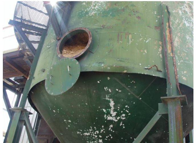
Photo ID No: 1190011_Photo_03_01_2012-010 Time: Approx. 14:15 Hatch for loosening sawdust on East side of sawdust storage silo for the Hurst Boiler. The camera is facing approx. SW.
