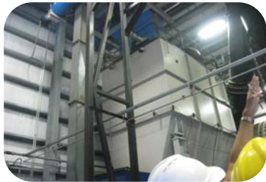
Biosolid Holding Hopper
