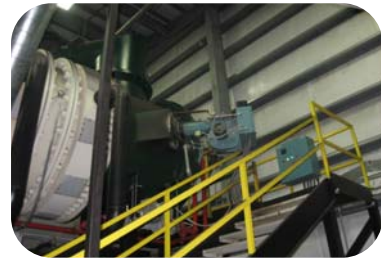
Start of the thermal oxidizer Syngas primary burner The white rings are the oxygen rings
