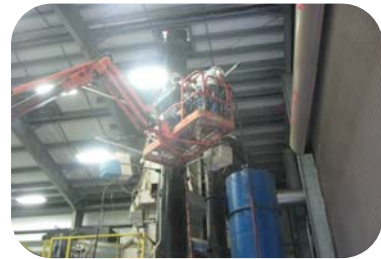
Stack test platform. Black tube is the exhaust stack Blue tank is the single pass wet scrubber
