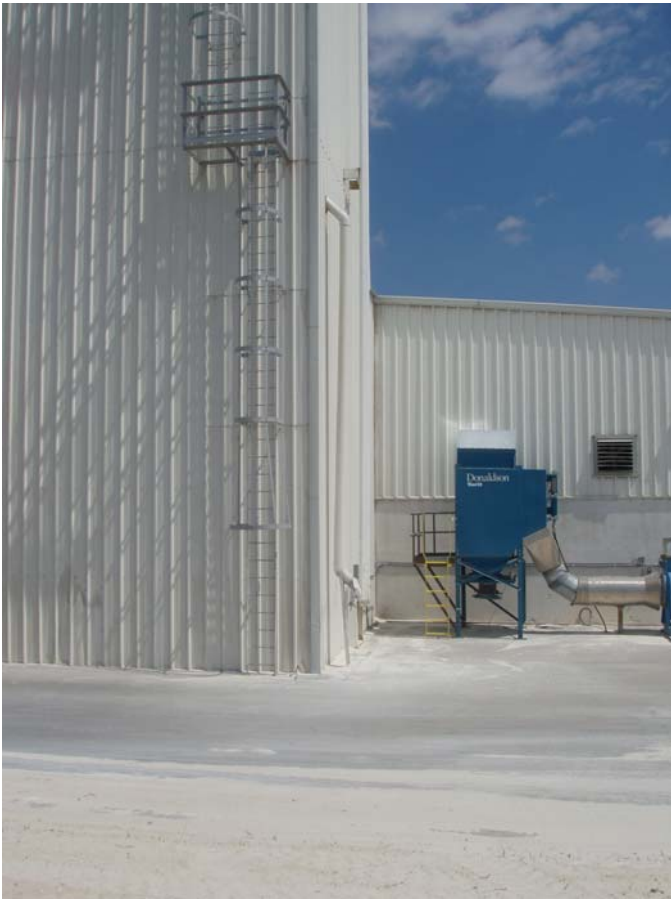
Photo ID No: 1050386_Photo_05_11_2012-018 Time: Approx. 11:30 AM View of new dust collector (not currently operating) and lower South and East sides of tower containing raw material storage bins. Camera is facing approx. N.
