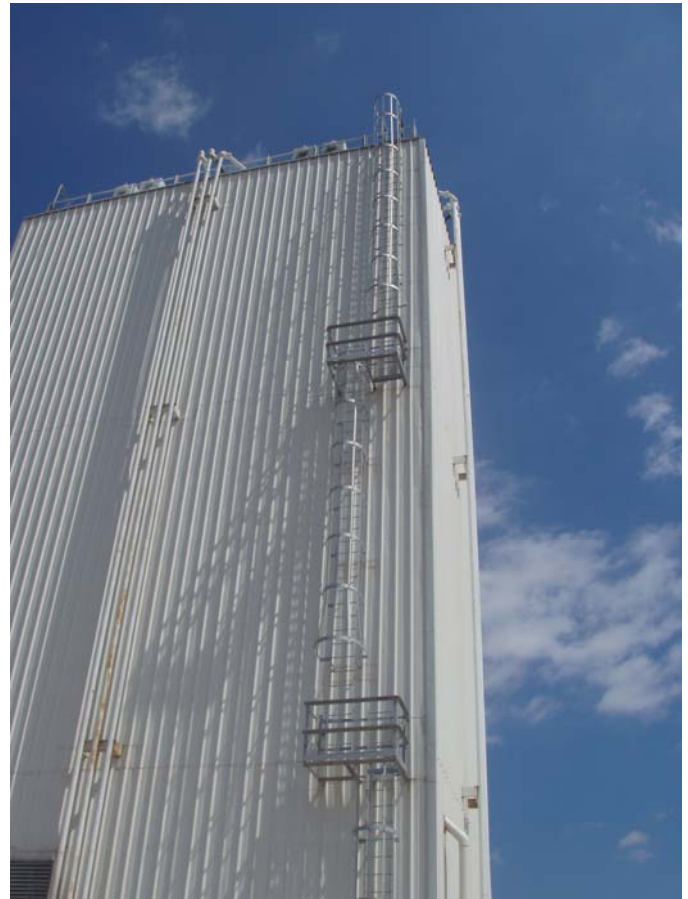
Photo ID No: 1050386_Photo_05_11_2012-019 Time: Approx. 11:30 AM View of upper South and East sides of tower containing raw material storage bins. Pipes, which are used for loading raw materials into raw material storage bins, are visible on the South and East sides of the building. Camera is facing approx. N.
