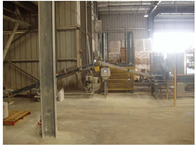
Photo ID No: 1050386_Photo_05_11_2012-006 Time: Approx. 10:45 AM Conveying equipment to send packaged material from packing machine to the machine that organizes the packaged materials onto pallets (not visible in this photograph). Camera is facing approx. W.
