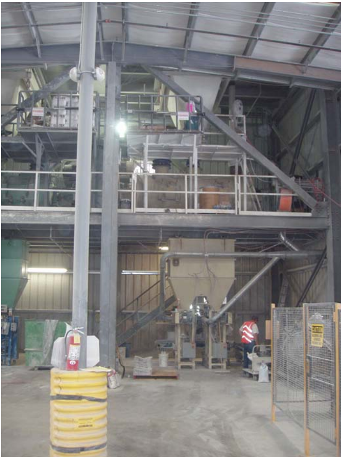
Photo ID No: 1050386_Photo_05_11_2012-002 Time: Approx. 10:45 AM View of original material processing equipment at facility. Camera is facing approx. S.
