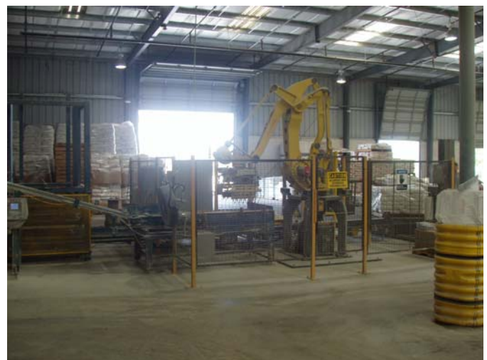
Photo ID No: 1050386_Photo_05_11_2012-007 Time: Approx. 11:00 AM Material organizing machine (yellow crane-like machine) that sorts material packages onto pallets. This machine is connected to the original material processing equipment at the facility. Camera is facing approx. NW.
