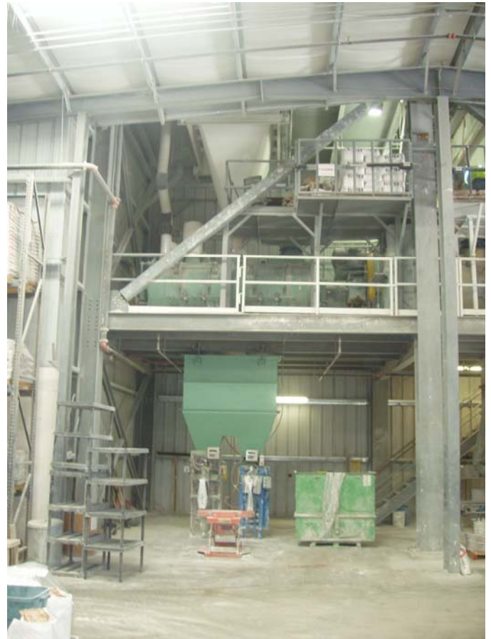
Photo ID No: 1050386_Photo_05_11_2012-010 Time: Approx. 11:00 AM View of new material processing equipment at facility. Camera is facing approx. S.
