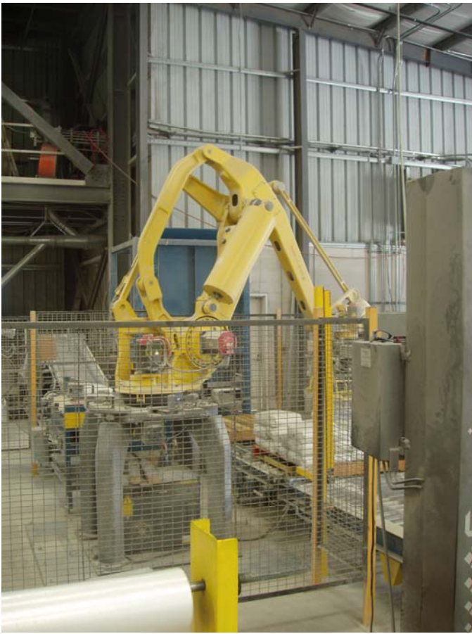
Photo ID No: 1050386_Photo_05_11_2012-013 Time: Approx. 11:00 AM View of machine for organizing material onto pallets. Camera is facing approx. SW.
