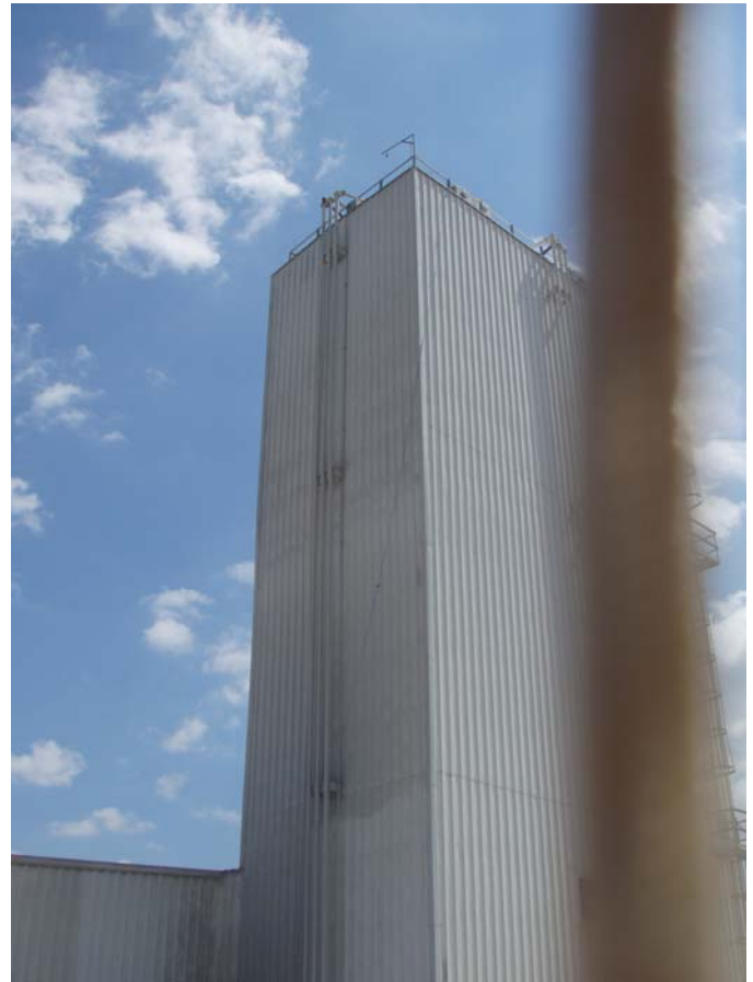
Photo ID No: 1050386_Photo_05_11_2012-015 Time: Approx 11:15 AM Exterior view of upper West and South sides of tower that contains the nine (9) raw material storage bins. Pipes, which are used to load raw materials into raw material storage bins, are visible on the South and West sides of the building. Bin vents are on top of tower (not visible in photo) and material processing equipment is inside on the bottom of the tower (inside building, not visible in photo). The blurry line in the foreground of the photograph (right side of photo) is the camera strap. Camera is facing approx. NE.
