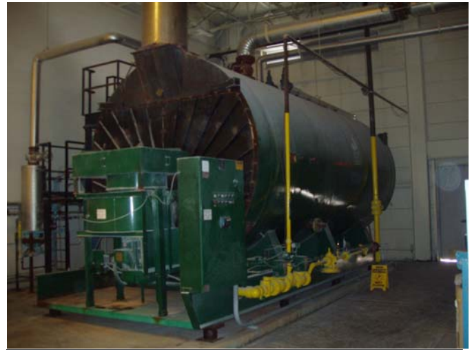
Photo ID No: 1050276_Photo_05_10_2012-012 Time: Approx. 11:30 AM The Johnston boiler, exempt from air operating permitting, supplies steam to the autoclaves at the facility. The camera is facing approx. SE.
