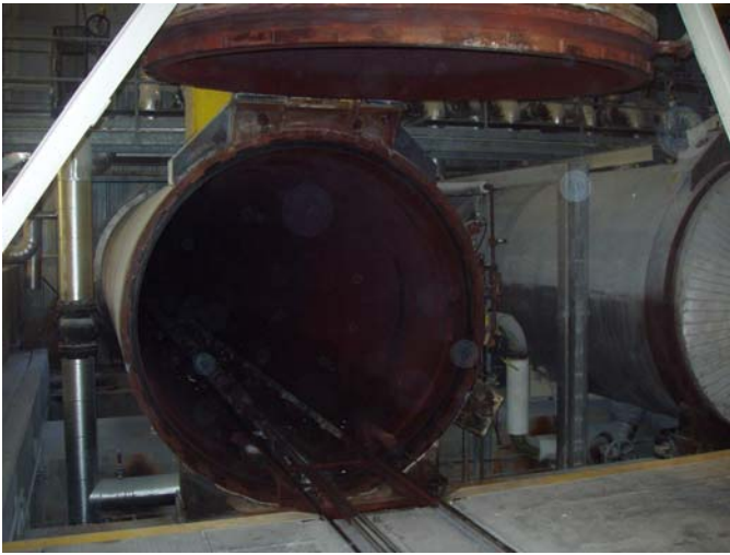
Photo ID No: 1050276_Photo_05_10_2012-010 Time: Approx. 11:15 AM Easternmost autoclave in building. Autoclave is open. The camera is facing approx. S.
