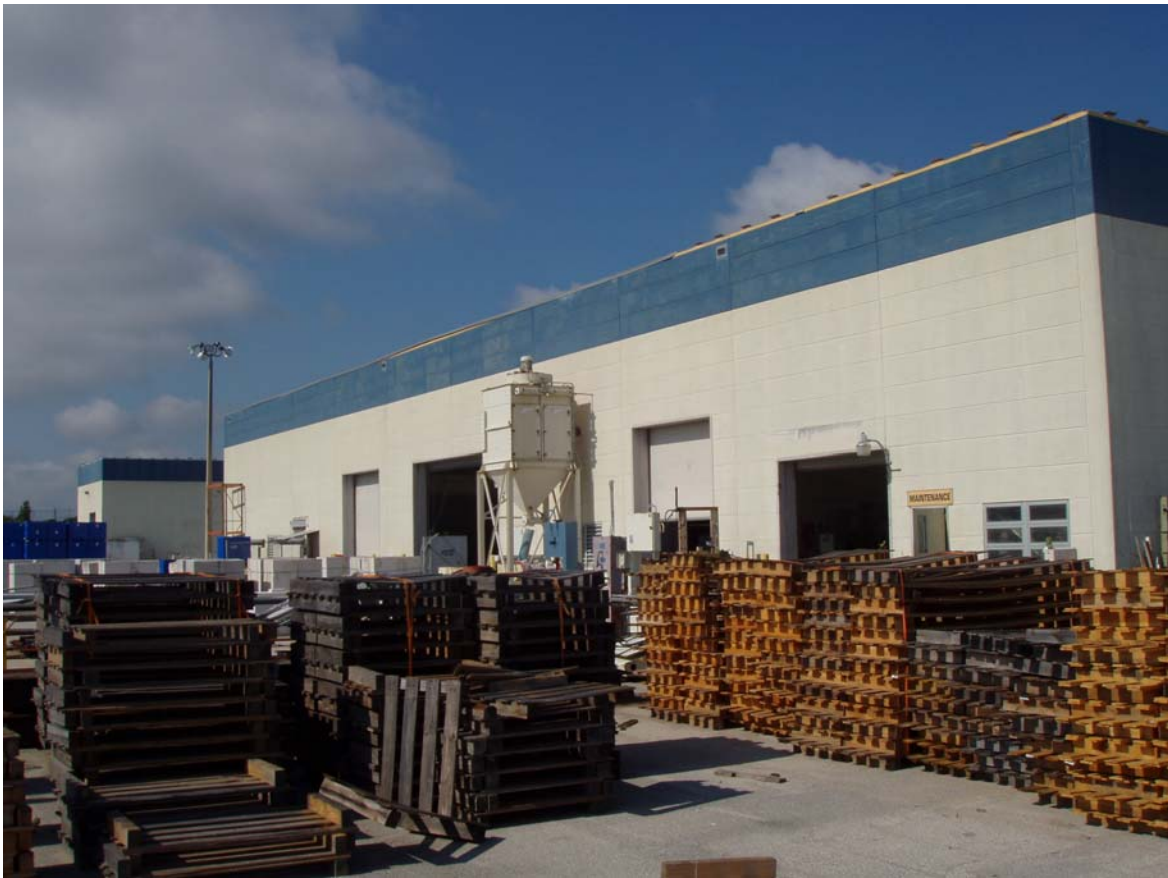
Photo ID No: 1050276_Photo_05_10_2012-003 Time: Approx. 09:45 AM The HANDTE Model PF 12-120 cartridge filter baghouse, visible on the center of the face of the building containing the cutting area, controls particulate matter emissions from the cutting area (EU007). The camera is facing approx. SW.
