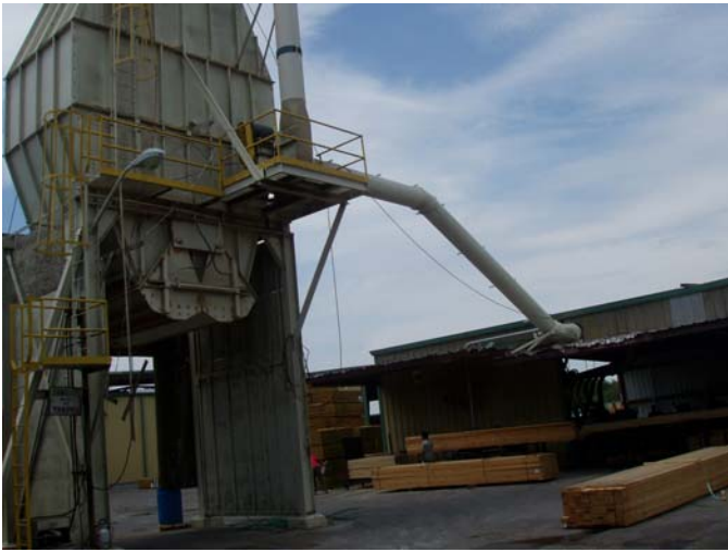
Photo ID No: 1050244_05_15_2012-012 Time: Approx. 12:15 PM Sawdust storage bin with main dust pickup line. The camera is facing approx. SW.
