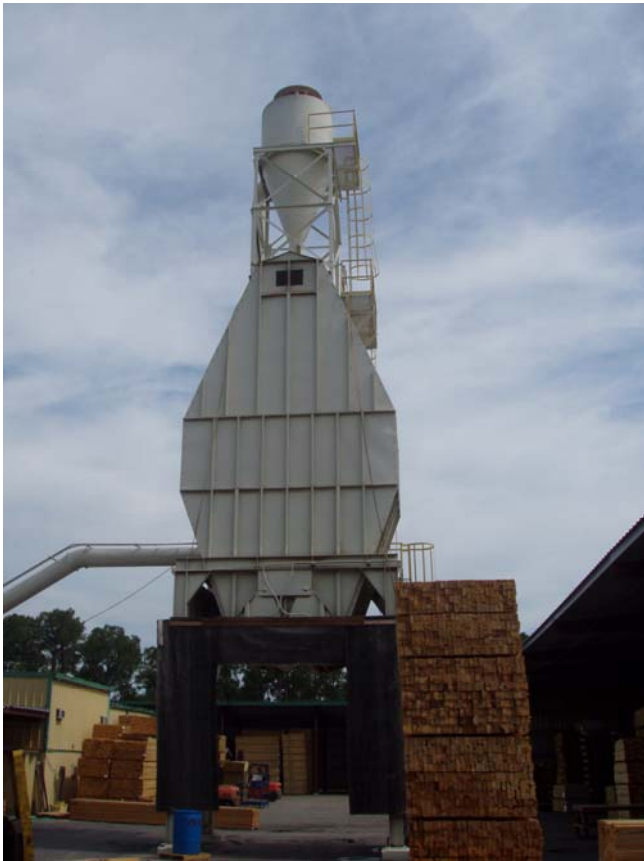
Photo ID No: 1050244_Photo_05_15_2012-003 Time: Approx. 10:45 AM A U.S. Metal Works, Inc., 7' diameter cyclone separator is installed on top of the 20 unit sawdust storage bin at this facility, which is visible in this photograph. The cyclone controls particulate matter (PM) from dust pickup points that send sawdust from sawing operations at the facility to the sawdust storage bin. The camera is facing approx. N.
