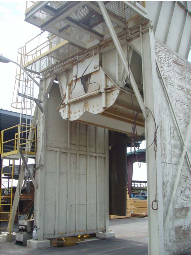
Photo ID No: 1050244_Photo_05_15_2012-010 Time: Approx. 12:15 PM Opening of the sawdust storage bin. The camera is facing approx. SE.
