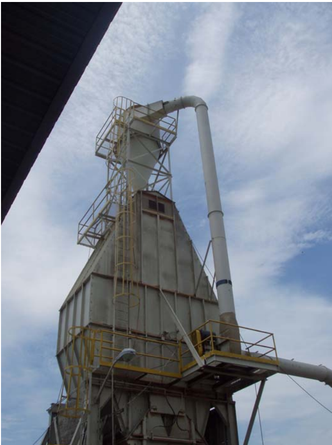
Photo ID No: 1050244_Photo_05_15_2012-013 Time: Approx. 12:15 PM Sawdust storage bin with main dust pickup line and line leading to cyclone. The camera is facing approx. SW.
