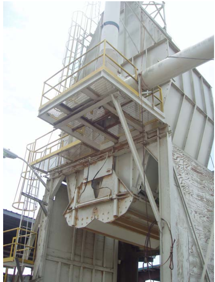
Photo ID No: 1050244_Photo_05_15_2012-011 Time: Approx. 12:15 PM View of the opening of the sawdust storage bin and of the main dust pickup line. The camera is facing approx. SE.
