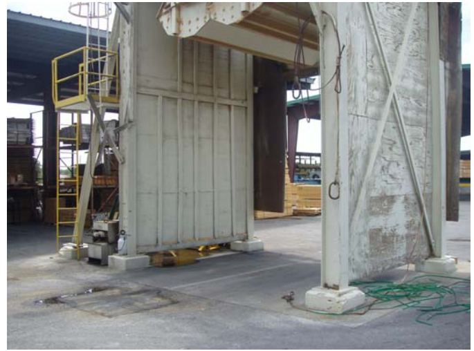
Photo ID No: 1050244_Photo_05_15_2012-009 Time: Approx. 12:15 PM Truck loading area for sawdust loading from sawdust storage bin. The camera is facing approx. SE.
