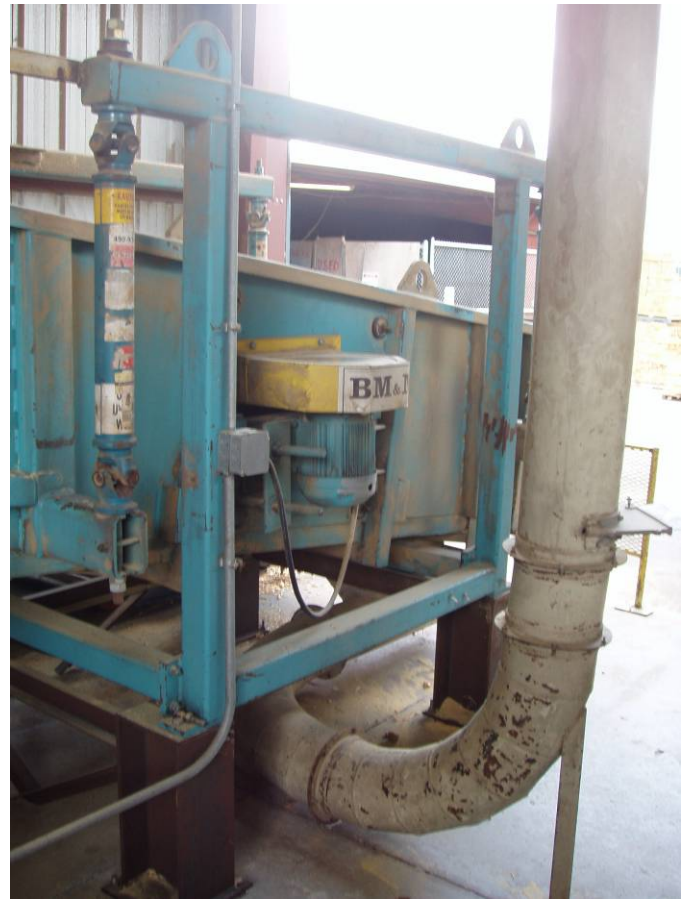
Photo ID No: 1050128_Photo_03_29_2012-007 Time: Approx. 12:15 PM View of dust pickup point (vertical pipe with curved bottom) for picking up dust from the bottom of the screener for wood chips, located after exit of hammer hog. The screener screens out small particles. The camera is facing approx. NW.
