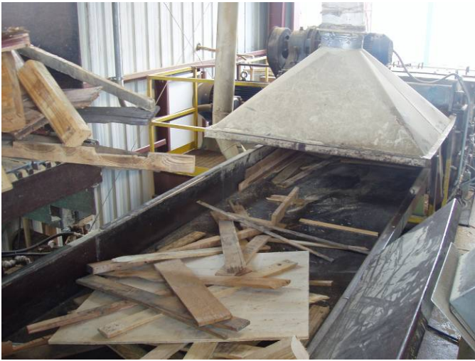
Photo ID No: 1050128_Photo_03_29_2012-008 Time: Approx. 12:15 PM Close-up photo of the mechanical shaking pad with wood waste leading to hammer hog. The hood for picking up dust, prior to wood waste entering the hammer hog, is visible over the mechanical shaking pad. The camera is facing approx. SE.
