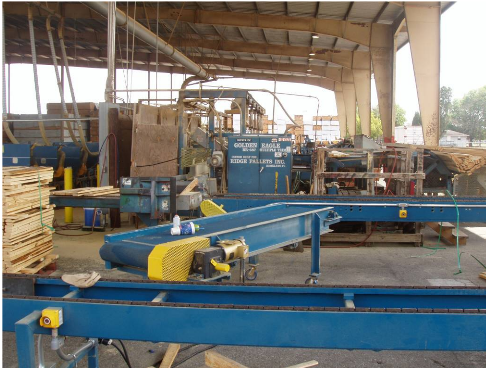
Photo ID No: 1050128_Photo_03_29_2012-014 Time: Approx. 12:30 PM Sawing equipment in the Big Shed at the facility. The camera is facing approx. E.
