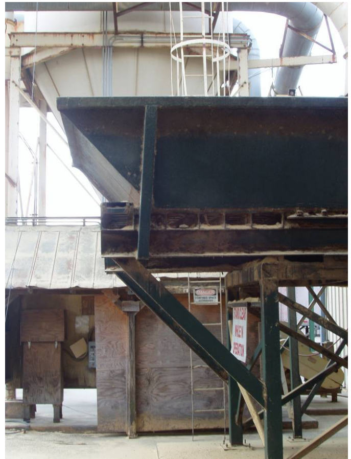
Photo ID No: 1050128_Photo_03_29_2012-005 Time: Approx. 12:15 PM Loading area with green loading bin for hammer hog. The central baghouse for the facility is shown in the background of the photo. The camera is facing approx. S.
