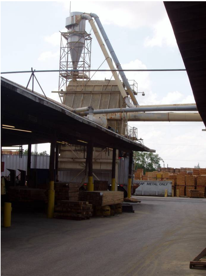
Photo ID No: 1050128_Photo_03_29_2012-002 Time: Approx. 12:00 PM View of cyclone on top of sawdust truck loading area. In the foreground of the photo, the small East cutting shed is visible. The camera is facing approx. SSE.
