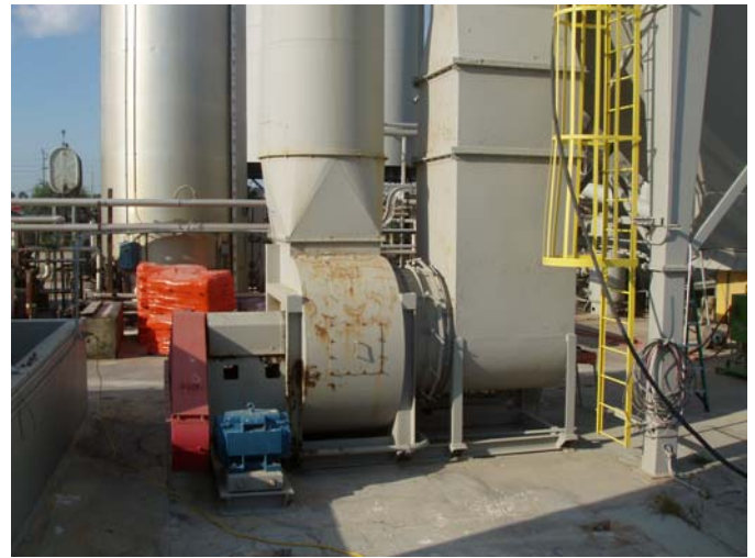
Photo ID No: 1010027_Photo_04_10_2012-004 Time: Approx. 09:30 AM View of stack, base portion. The camera is facing approx. SW. The height of the stack is approximately 30 feet.
