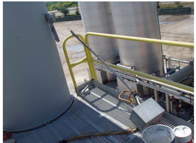
Photo ID No: 1010027_Photo_04_10_2012-012 Time: Approx. 11:00 AM View of the probe after stack test run #2. The camera is facing approx. SE.
