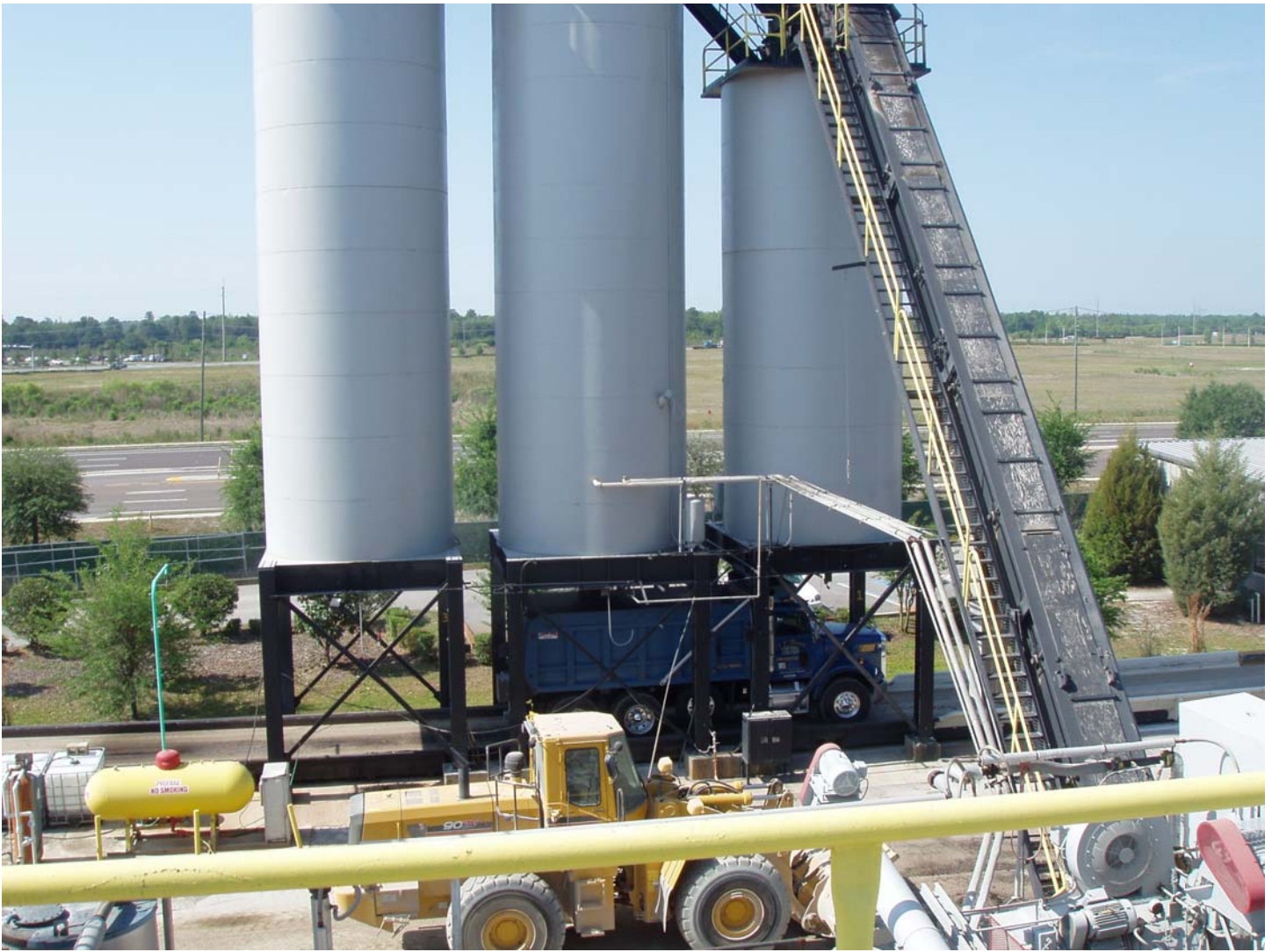
Photo ID No: 1010027_Photo_04_10_2012-018 Time: Approx. 11:00 AM Asphalt storage silos. Truck loadout was occurring during the end of the compliance inspection (truck is visible beneath silos). The camera is facing approx. SW.
