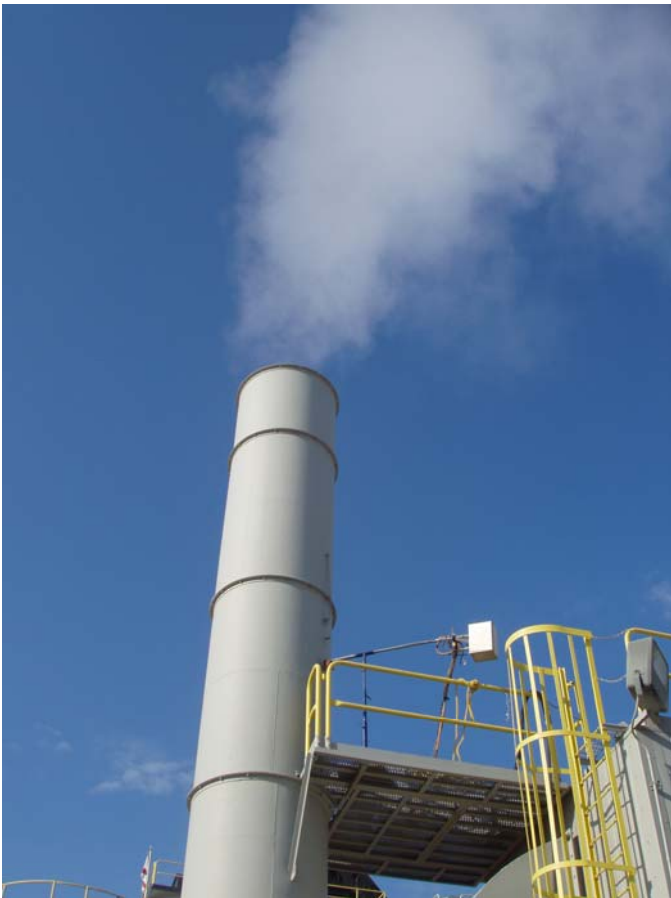
Photo ID No: 1010027_Photo_04_10_2012-010 Time: Approx. 10:15 AM Photo taken near the end time of stack test run #2. The camera is facing approx. SW.
