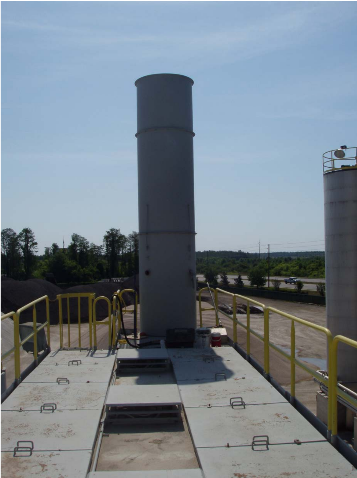
Photo ID No: 1010027_Photo_04_10_2012-015 Time: Approx. 11:00 AM View of top of stack and stack testing equipment, shortly after stack test run #2. The camera is facing approx. E.
