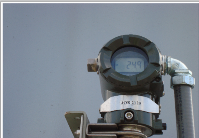
Photo 3: Digital gauge showing -24.9 vacuum near the blower within the collection system
