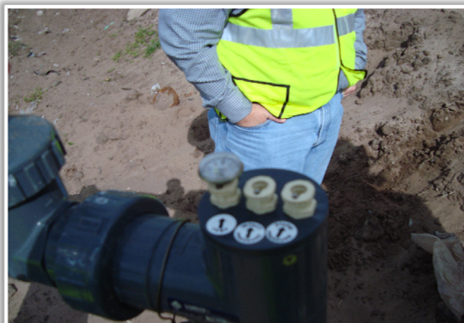
Photo 12: Top of typical well showing temperature point (left), impact point (center) and static vacuum point (right). The thermometer is removable for reading. Liner, cover soil and sod is yet to be placed.
