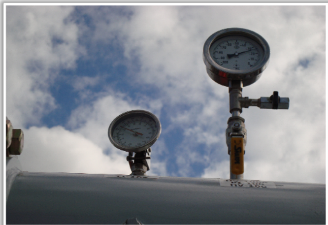
Photo 4: Needle gauges on inlet to blowers show temperature (left) and vacuum (right) within the collection system. Inlet pressure can be set so that collection system well adjustments and weather fronts have no pressure effects.
