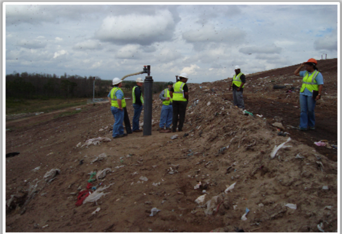
Photo 14: North view of a typical well. Gas collection system and flare are in background. Liner, soil and sod yet to be placed.
