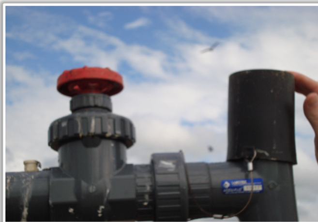
Photo 10: Top of well #007 showing black cover(right) in place that is removed and hanging down in photo 9. Red valve (middle) enables temperature/air adjustments. White connection (left) enables header pressure measurements. This same configuration is used on all gas collection wells.
