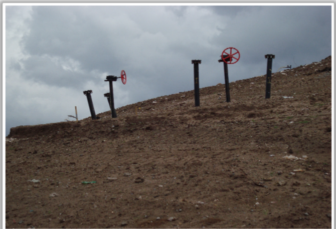
Photo 16: ENE view of gas isolation valves located near collection system.
