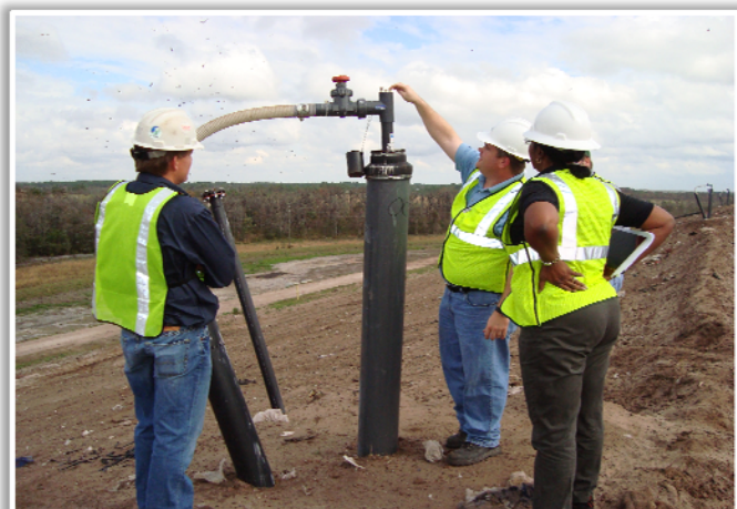
Photo 9: Gas collection well #007 in area at final grade. Liner, cover soil and sod is yet to be placed. Pitot tubes are installed in all the wells.
