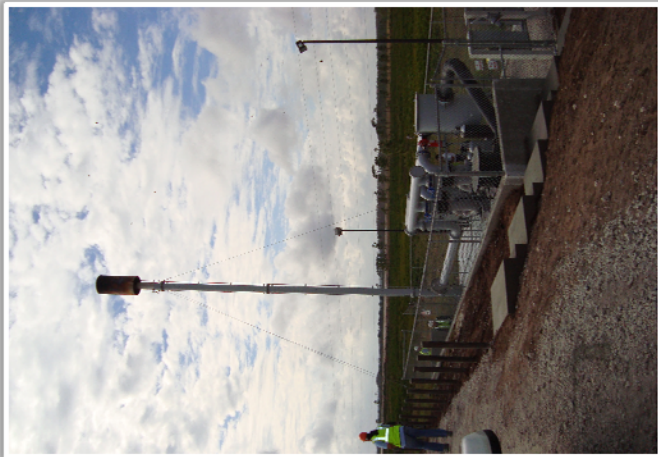
Photo 1: SSW view of landfill gas collection and control device.
