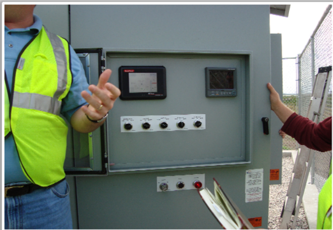
Photo 5: Open collection system control panel.
