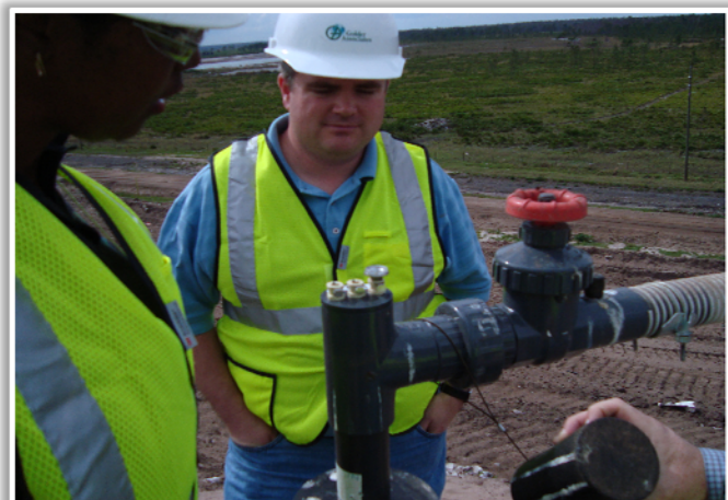
Photo 11: Top of typical well showing monitoring points (center of photo) located under removed black cover. Liner, cover soil and sod is yet to be placed.
