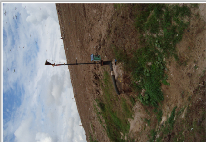
Photo 15: NNE view of leachate odor control station used before collection and control system became operational.
