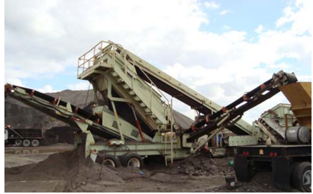
Screener and four (4) conveyor belts.
