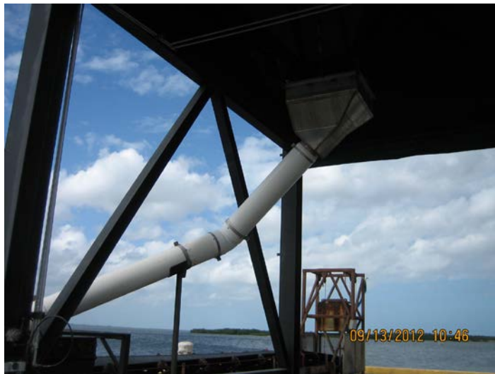
Photo ID No: IMG_431—Emission Unit No. 013 for Ship Unloading to Storage (New Hopper).
