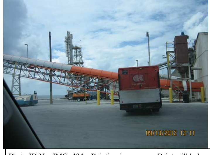
Photo ID No: IMG_434—Painting in progress. Paint will help protect conveyor covers from the elements.
