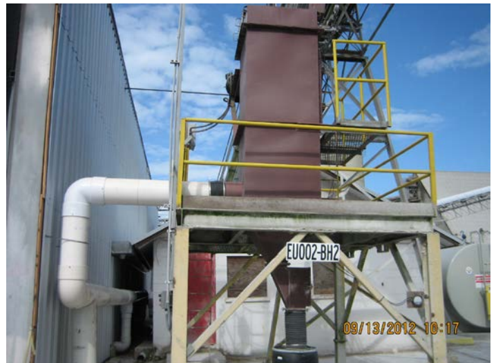
Photo ID No: IMG_428—Baghouse 2 (Emission Unit No. 002) for Railcar Unloading Building.
