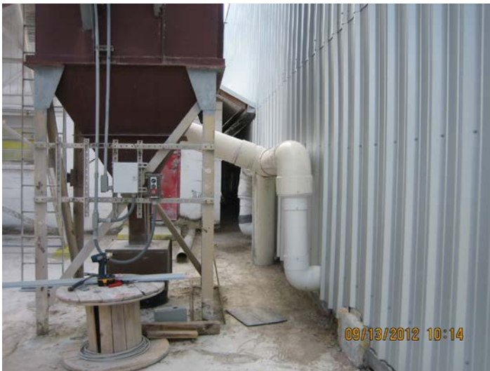
Photo ID No: IMG_426—Baghouse 3 (Emission Unit No. 003) for Railcar Unloading Building.
