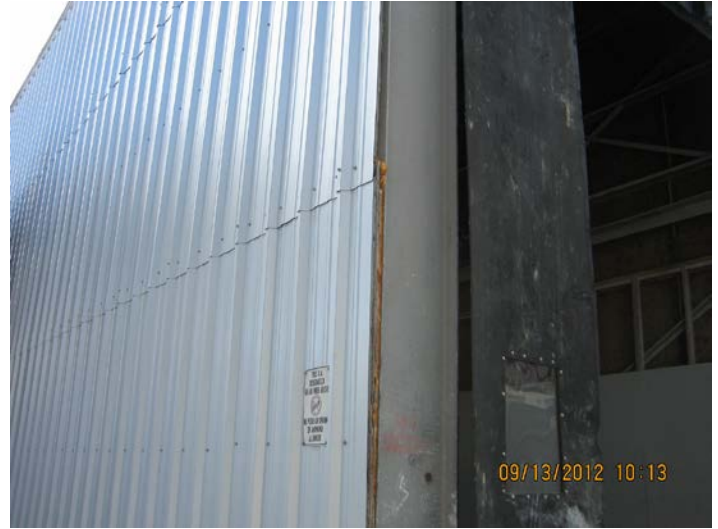
Photo ID No: IMG_425--This photos documents new aluminum skin on the Railcar Unloading Building.
