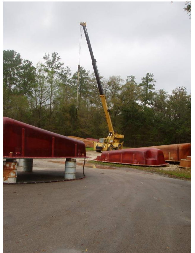
Photo ID No: Photo_0530363_02_23_2012-8 Time – Approx. 11:00 AM Crane used to lift each finished pool out of its mold. The camera is facing approx. NNW.
