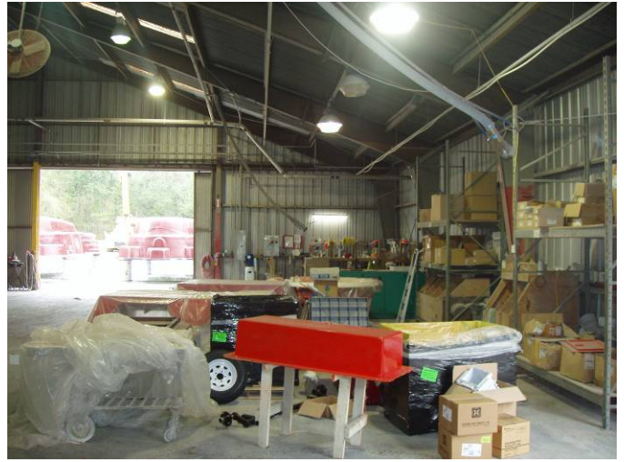
Photo ID No: Photo_0530363_02_23_2012-11 Time – Approx. 11:15 AM Another view of the mold repair area in the building. The camera is facing approx. N.
