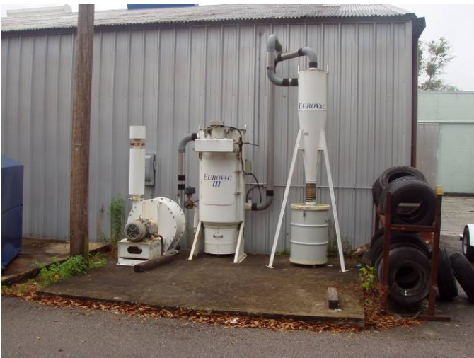
Photo ID No: Photo_0530363_02_23_2012-6 Time – Approx. 11:00 AM The Eurovac III system uses filters to capture and collect dust from tools and operations within the building. The camera is facing approx. WSW.
