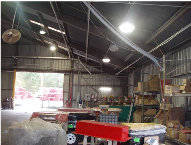
Photo ID No: Photo_0530363_02_23_2012-10 Time – Approx. 11:15 AM Pool molds are repaired and maintained on this side, the East side, of the building. Vacuum connections for the Eurovac III system, which uses filters to capture and collect dust from tools and operations within the building, are visible in this photograph. One of these vacuum connections is visible in the foreground of this photograph, which is the grey cable diagonally. The camera is facing approx. N.
