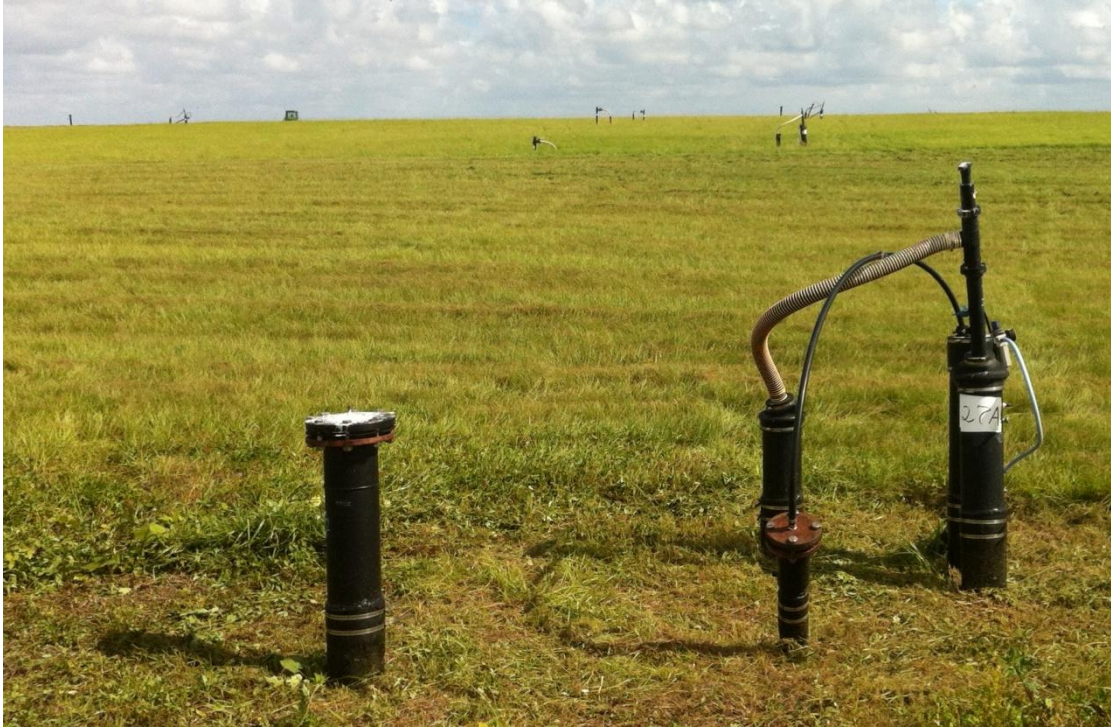
Cell 2 Monitoring Well 27A. More wells in the background
