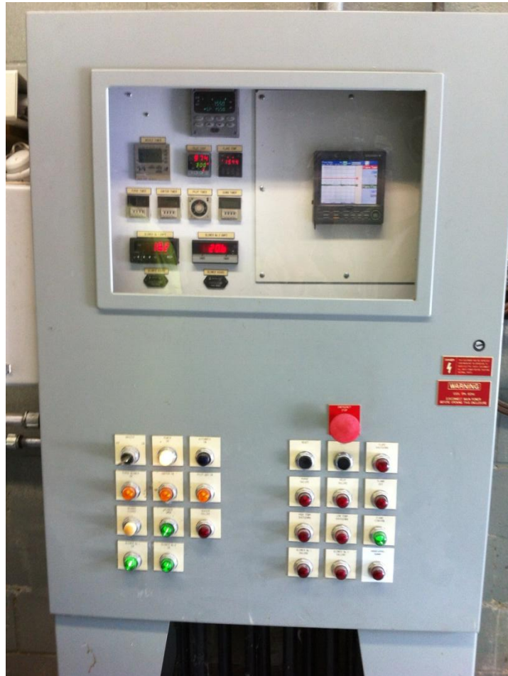
Control Panel with gas flow/flare temperature monitoring/recorder
