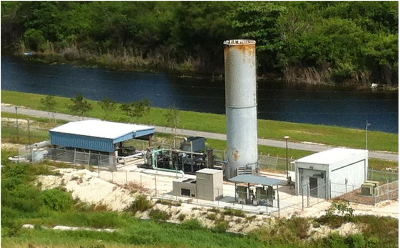
Flare (EU002) Station. Control Building to the right (east). New equipment for sending gas to the WWTP on the left (west) side.
