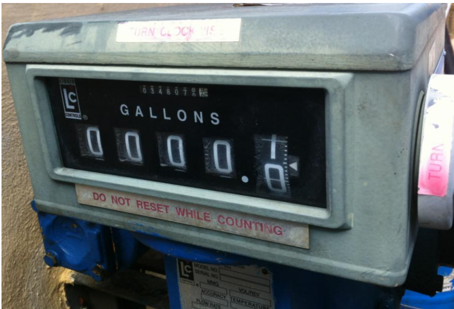
Diesel Fuel Meter
